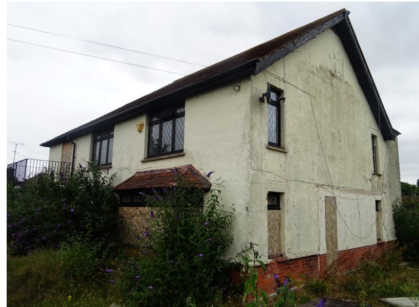
Figure 8: The Poor Condition of the Building
