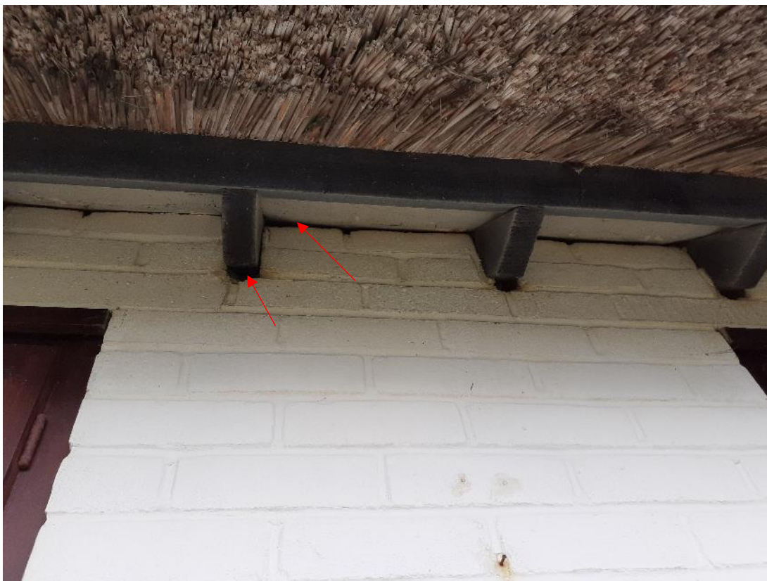
Photo 11: gaps under the eaves and under purlins on the southern facing elevation of the single storey extension.
