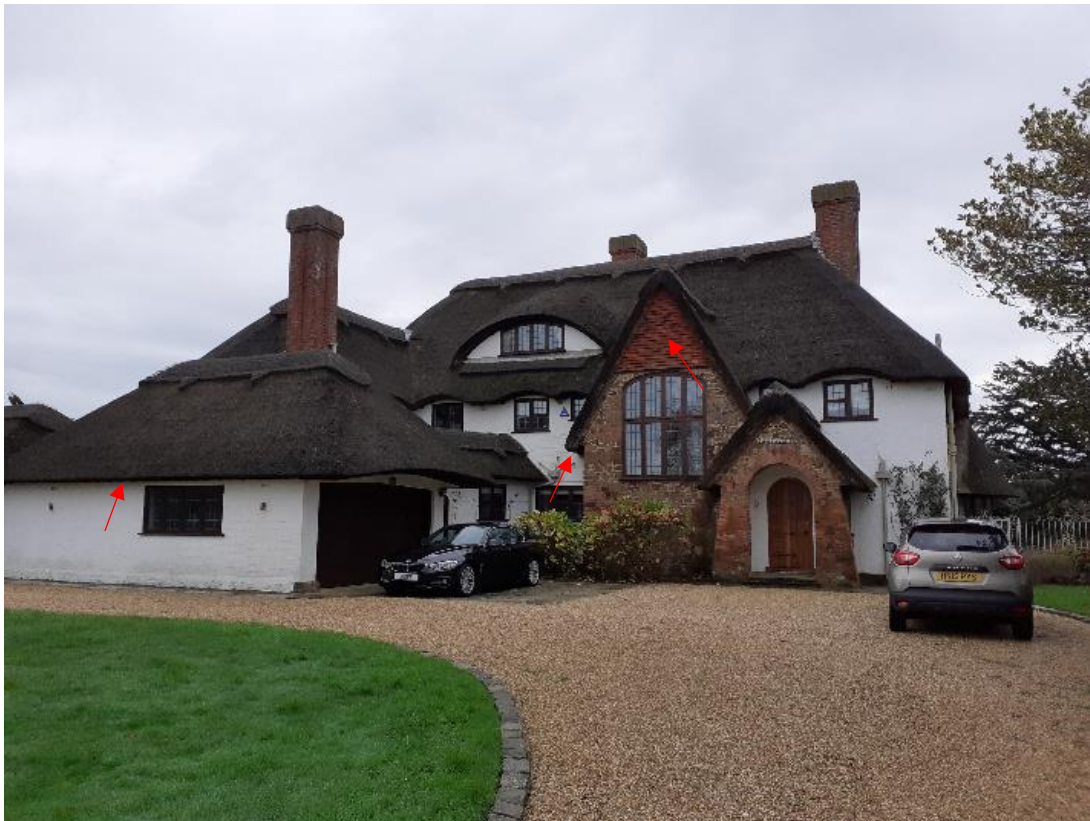
Photo 1: northern elevation of the building. Red arrows indicate location of suitable roosting crevices for bats.
