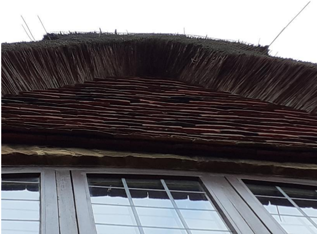
Photo 4: close up of gaps under hanging tiles on the northern gable end.
