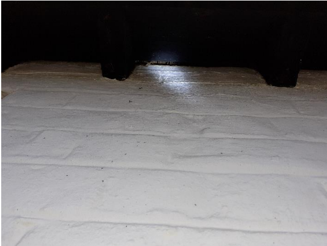
Photo 2: close up of gaps under the eaves running along the northern elevation of the single storey extension.
