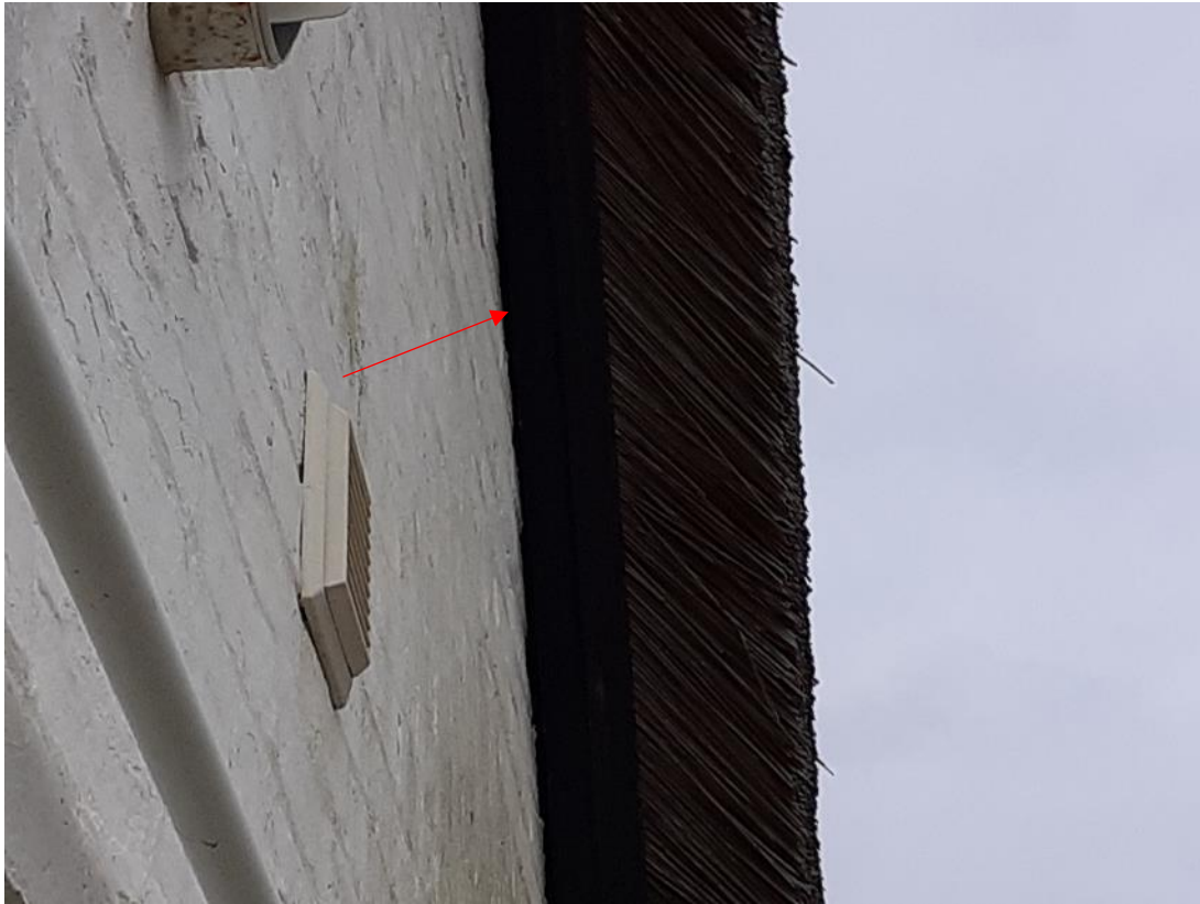
Photo 10: close up of gaps under the barge board on the eastern facing elevation of the two storey section.
