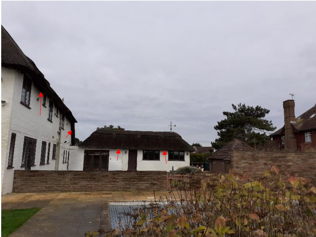
Photo 8: eastern and southern elevations of B1. Gaps are present along the lengths of the eaves on the two storey and single storey areas of the building and also under the barge boards along the northern edge.
