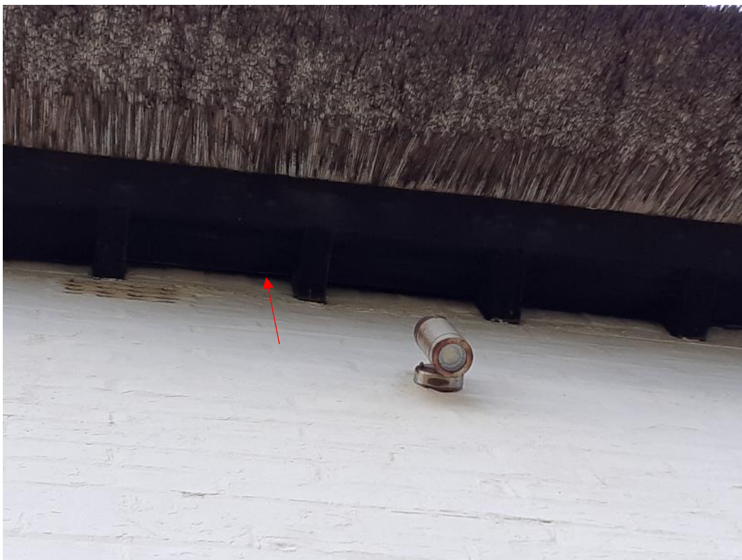
Photo 9: close up of gaps under the eaves on the eastern facing, two storey elevation.
