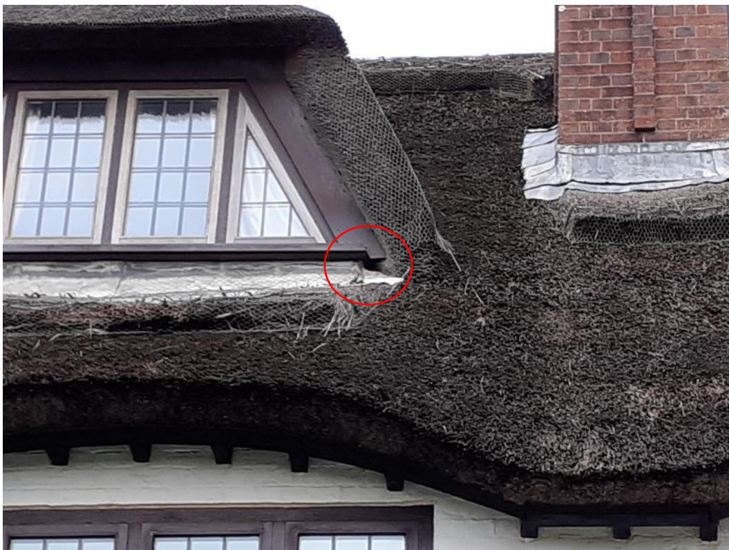
Photo 7: close up of gaps at the corner of the dormer window which could provide suitable roosting habitat for crevice dwelling bats.
