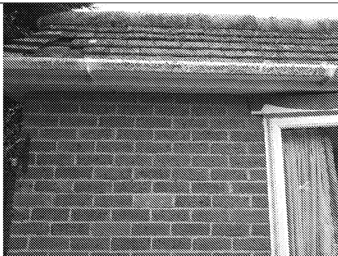
Photograph 4: Missing tiles on extension
