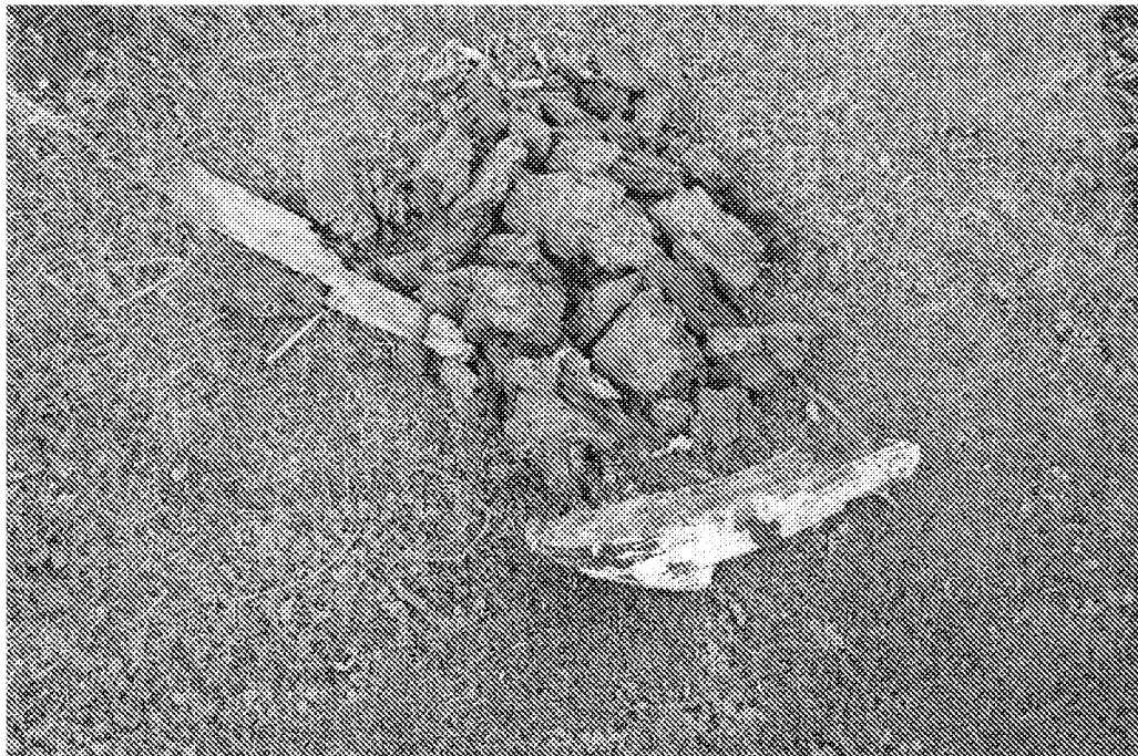
Fig 5 Loose decayed wood removed from inside cavity
