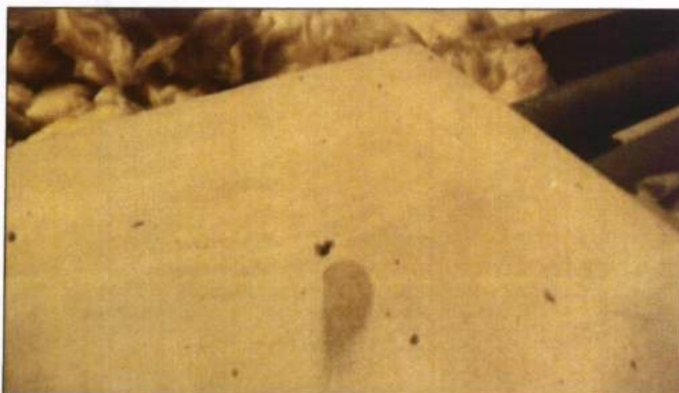
Photo 12: A few (c5) Old small bat dropping were located in the roof void.
