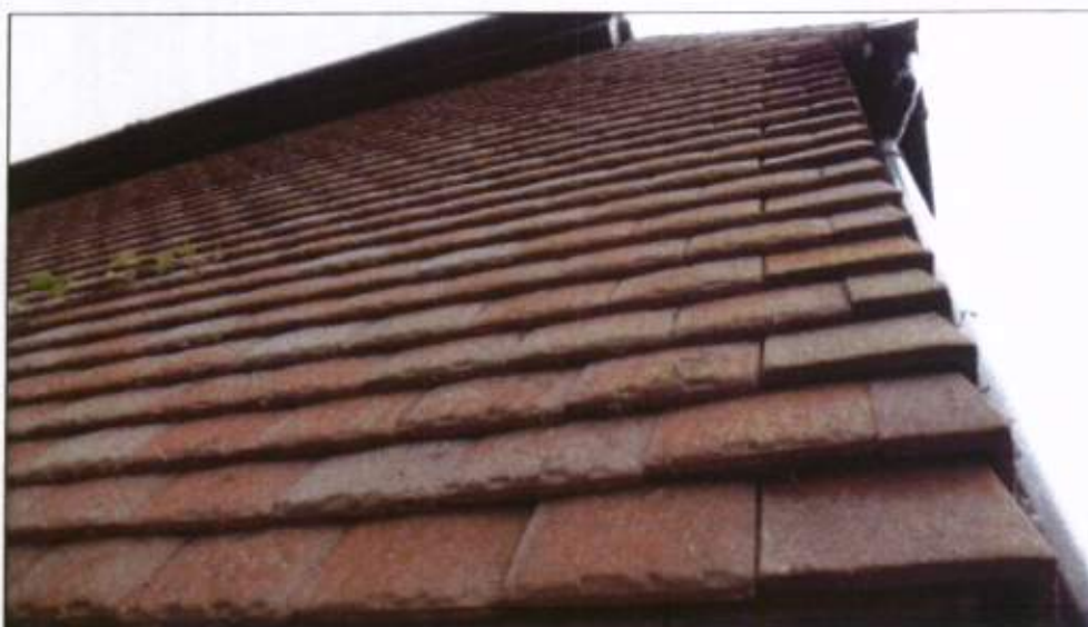
Photo 8: Hanging tiles are generally tightly fitting with few access opportunities
