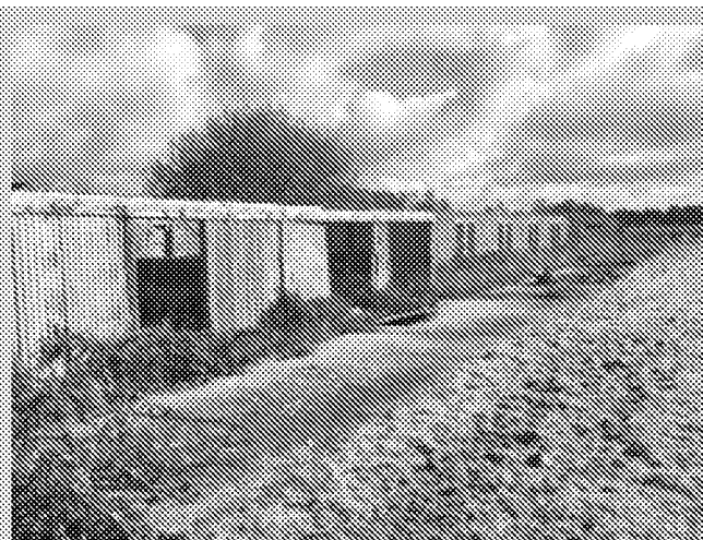
Photo 2: Derelict piggy runs and adjacent hard standing.
