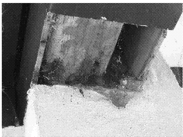
DSC02874 Rotted bearing end to timber beam
