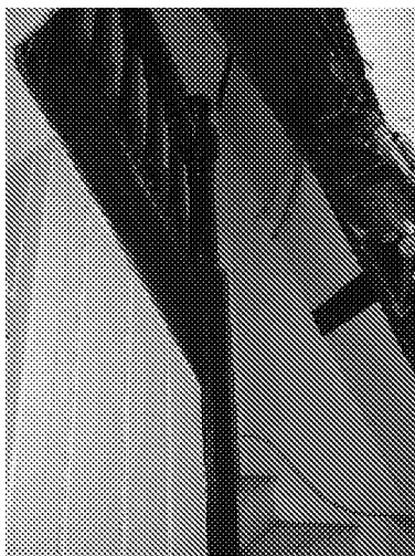
DSC02922 Inappropriate services
