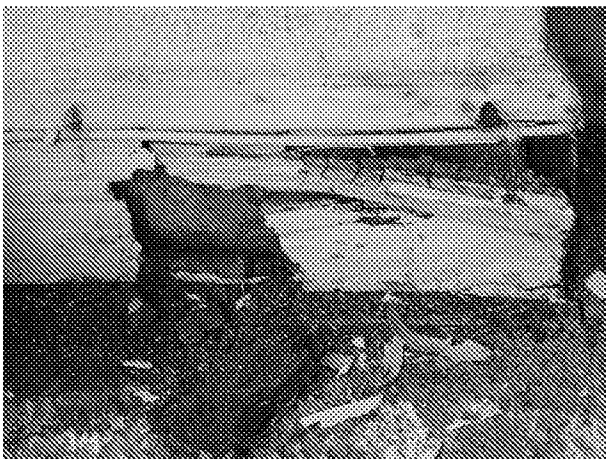
DSC02873 Dry rot in skirting
