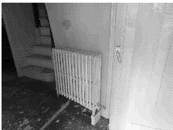
DSC02907 Cast iron radiator
