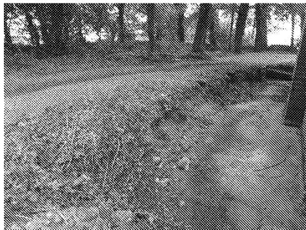
DSC03184 Exposed earth bank
