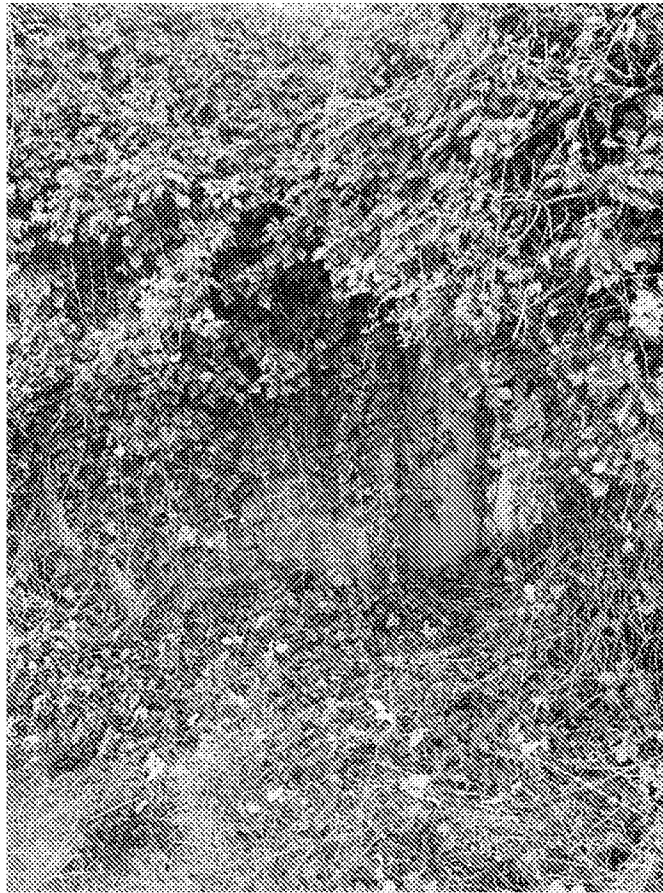
Figure 5.2 Building surrounded by overgrown vegetation.
