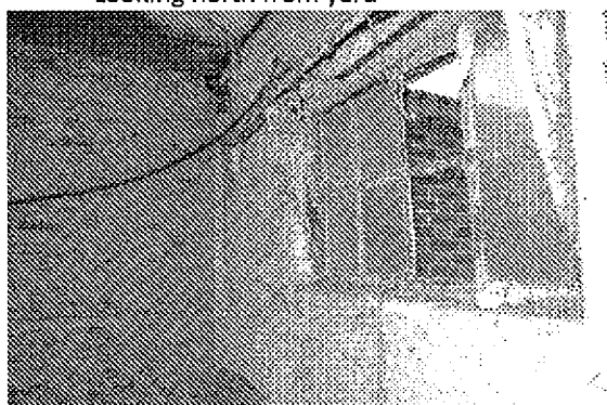
Missing window panes in stables, Building A
