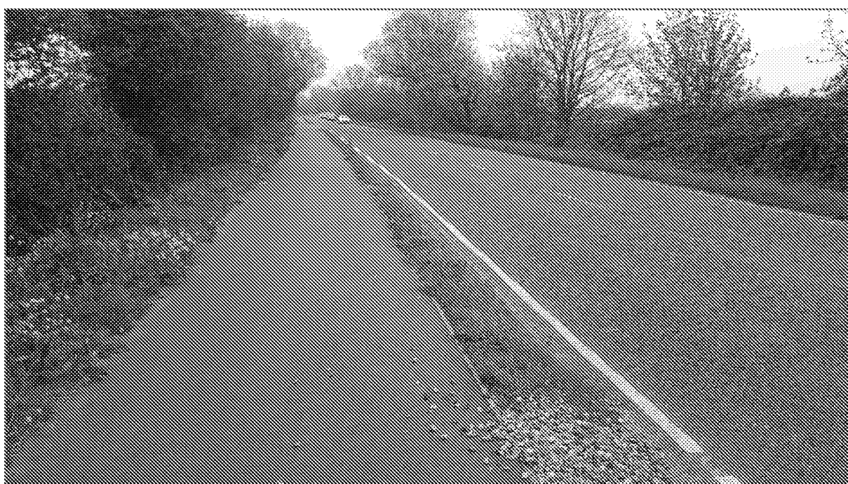
Photo 9 - Loose material on shared facility.
