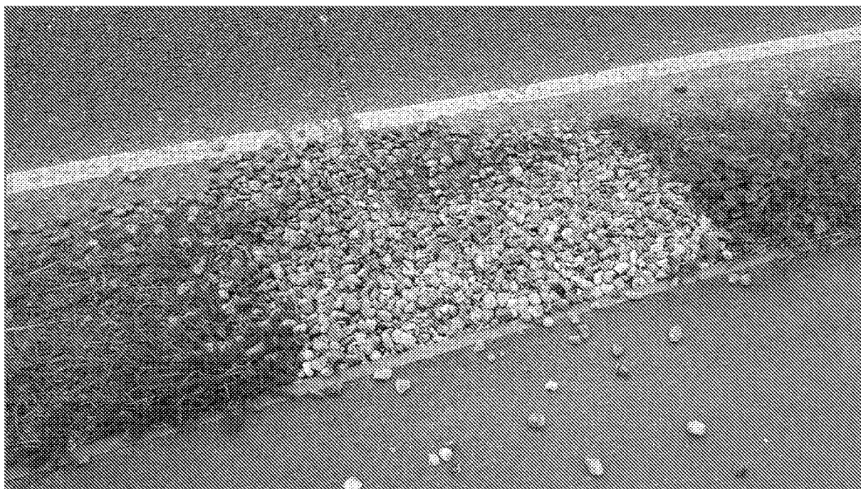
Photo 8 - Loose material adjacent to footway and highway.
