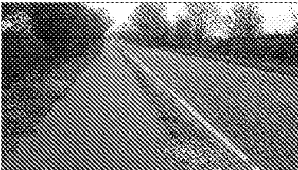
Photo 9 - Loose material on shared facility.
