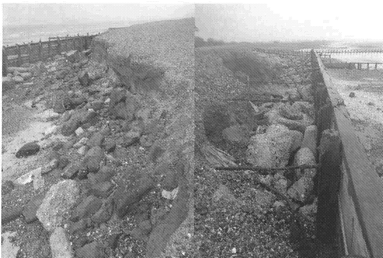
Figure 5-1 Damaged flood defences near Climping Beach (August 2018)
