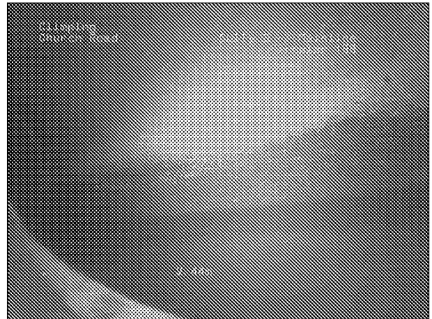
Photo: 54_3a 2.44m, Major connection without manhole
