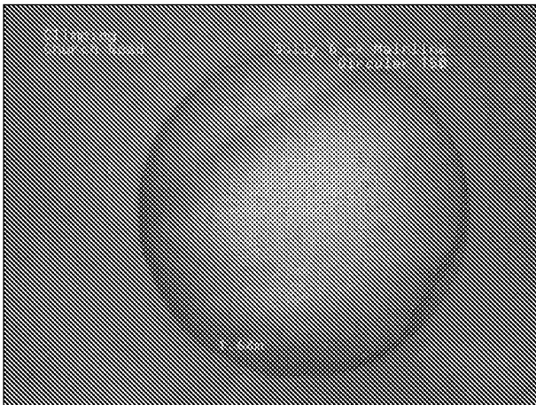
Photo: 58_4a 1.64m, Major connection without manhole
