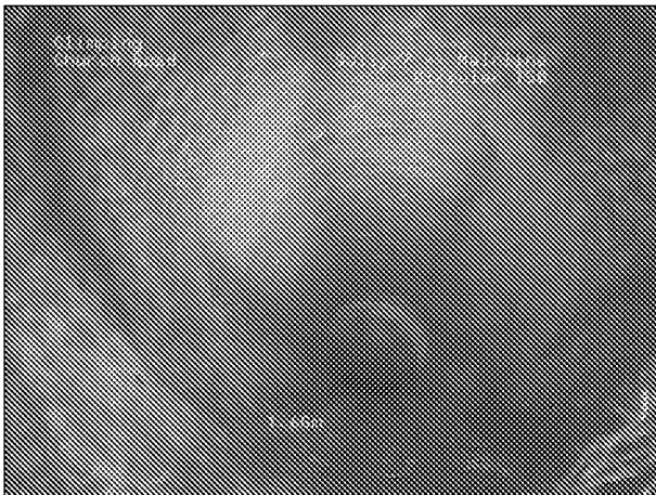
Photo: 84_4a 1.65m, Fine Roots at joint
