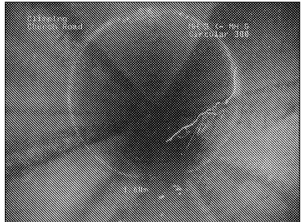
Photo: 68_4a 1.6m, Spalling at at 12 o'clock
