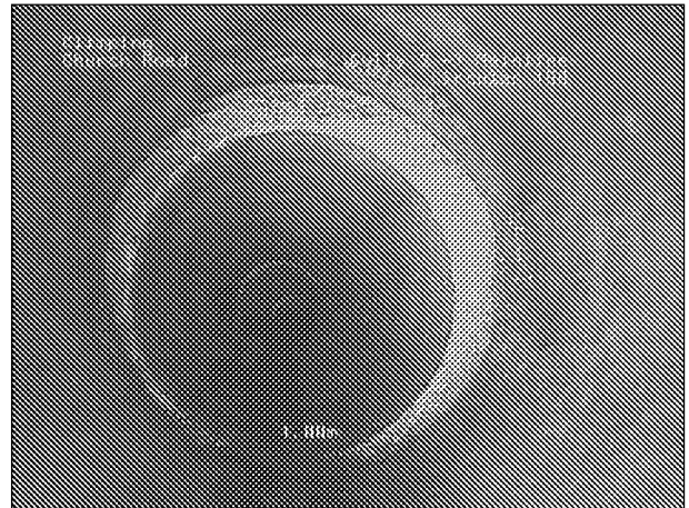
Photo: 38_3a 1.08m, Hole in sewer at joint from 12 to 02 o'clock
