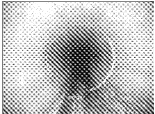
Photo: 127_12a 57.23m, Fine Roots at joint
