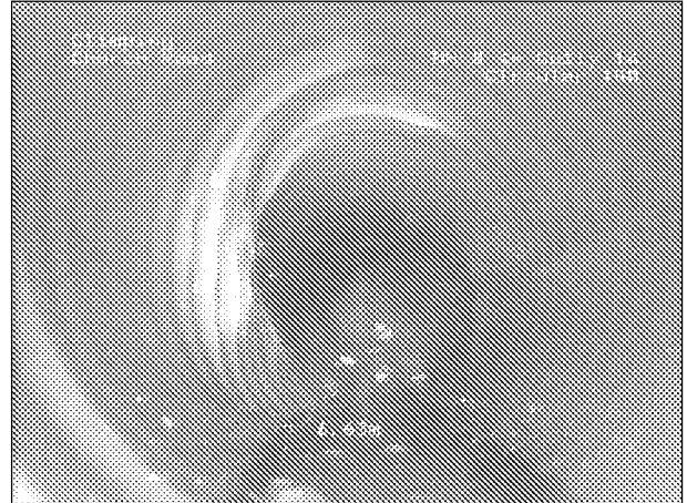
Photo: 103_3a 6.63m, Deformed drain/sewer 15 %
