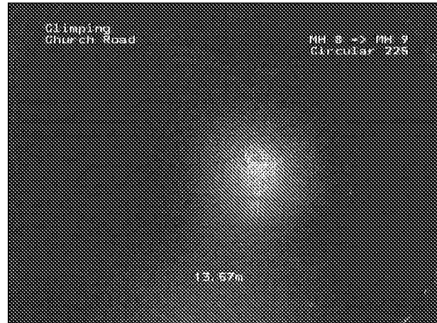
Photo: 115_3a 13.57m, Finish Node type, catchpit, reference number: MH 9
