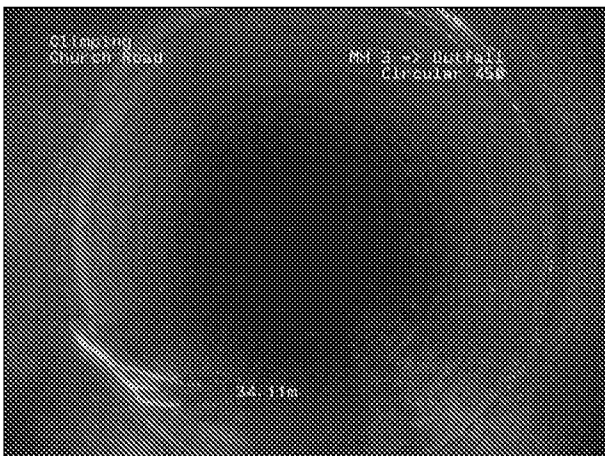
Photo: 79_6a 34.11m, Material of drain/sewer changes to Polyvinyl chloride
