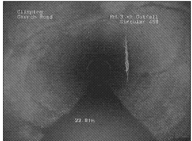
Photo: 78_5a 22.81m, Fractures multiple from 12 to 12 o'clock
