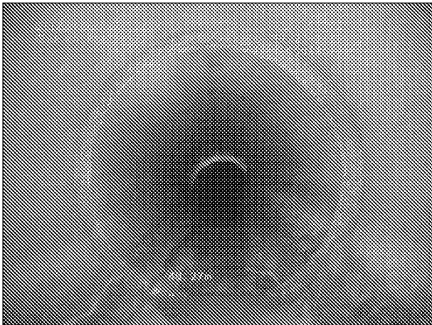
Photo: 27_14a 48.27m, Roots tap at joint
