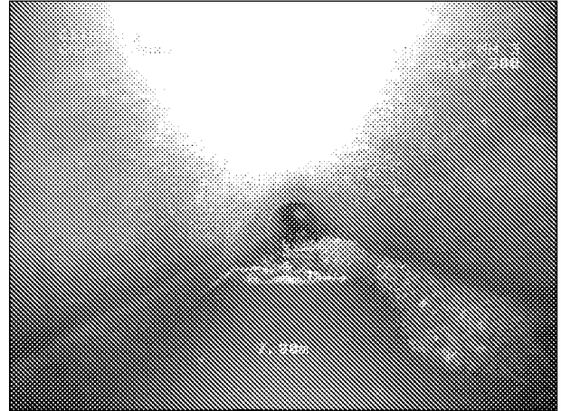
Photo: 100_3a 7.79m, Settled deposits fine 30 % cross-sectional area loss, Start
