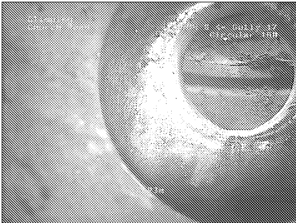
Photo: 112_3a 4.93m, Finish node type, gully, reference number: Gully 17
