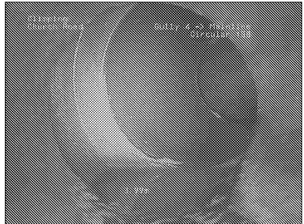
Photo: 50_4a 3.99m, Open joint large
