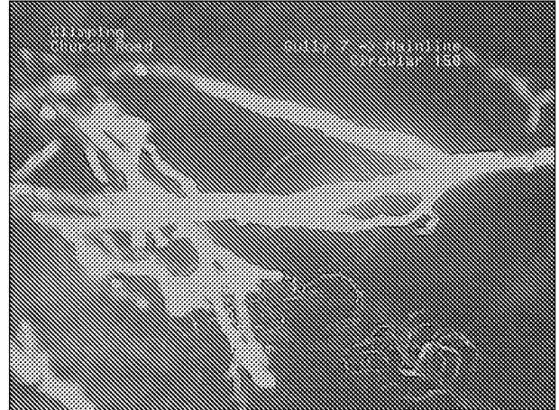
Photo: 83_3a 0.99m, Roots tap at joint
