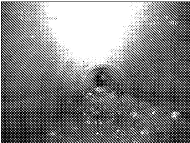
Photo: 15_4a 8.63m, Survey abandoned, Remark: Due to debris
