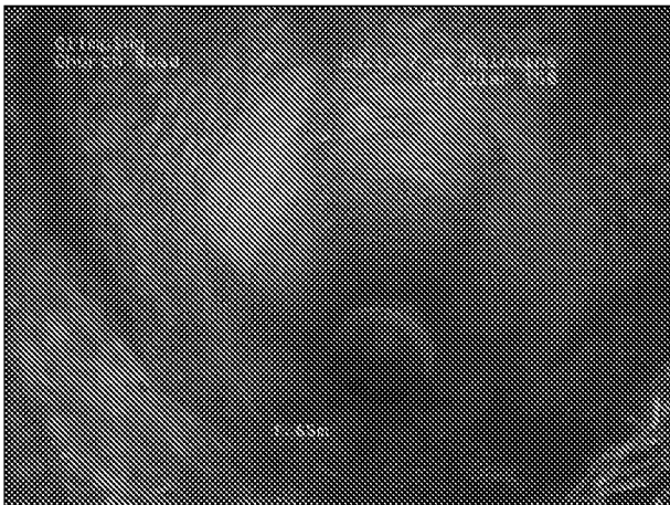
Photo: 84_4a 1.65m, Fine Roots at joint
