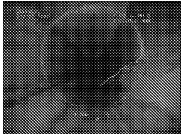
Photo: 68_4a 1.6m, Spalling at at 12 o'clock
