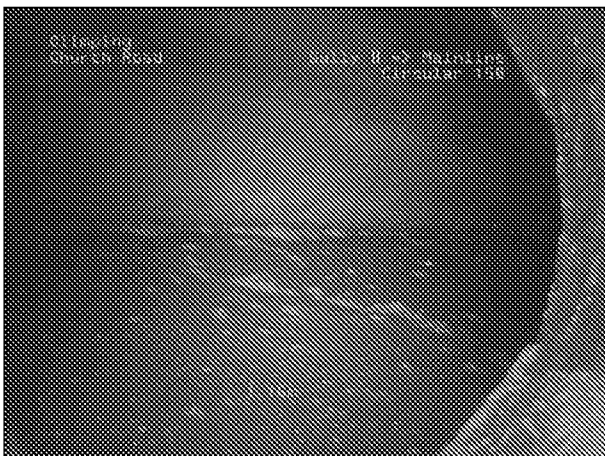
Photo: 91_4a 1.15m, Major connection without manhole
