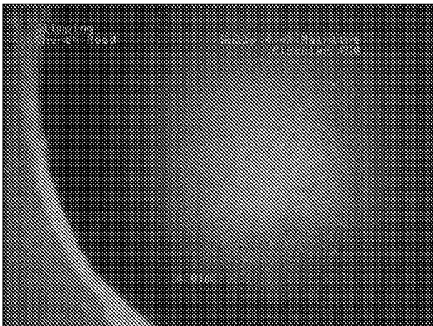
Photo: 51_5a 4.01m, Major connection without manhole
