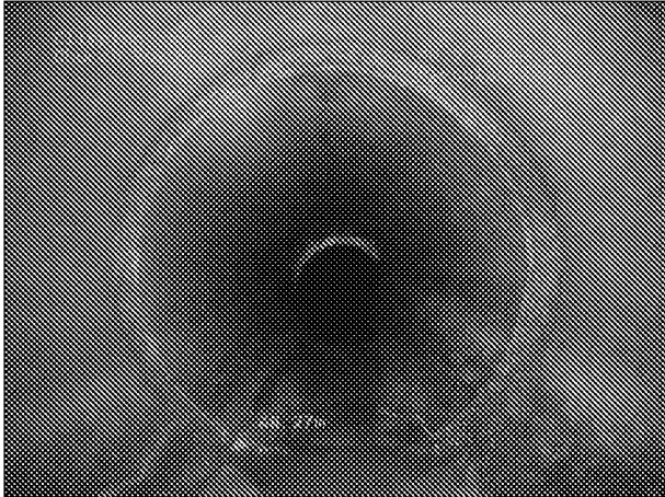
Photo: 27_14a 48.27m, Roots tap at joint
