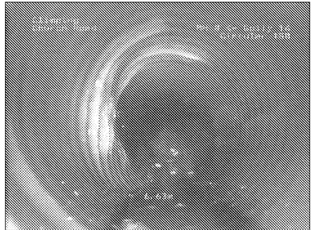
Photo: 103_3a 6.63m, Deformed drain/sewer 15 %
