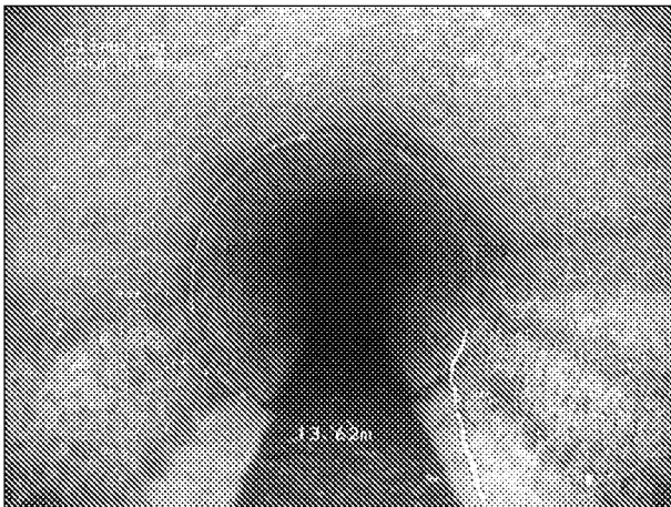
Photo: 120_5a 13.62m, Roots tap at joint
