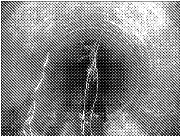
Photo: 123_8a 20.19m, Roots tap at joint
