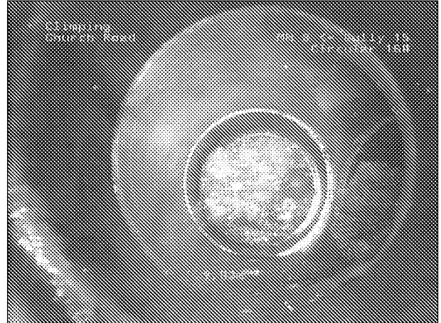
Photo: 107_3a 9.82m, Junction defective, connecting pipe is blocked at 03 o'clock, dia 150 mm
