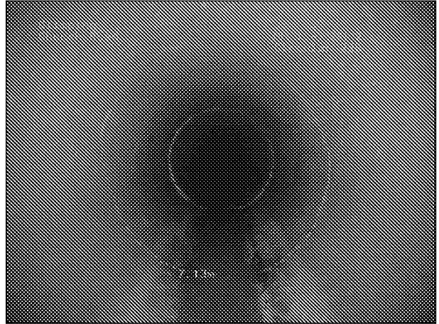
Photo: 6_3a 7.13m, Fracture Circumferential from 12 to 12 o'clock
