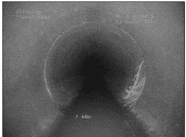
Photo: 18_5a 7.6m, Roots tap at joint
