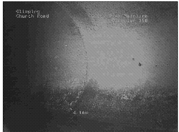
Photo: 41_6a 4.16m, Major connection without manhole
