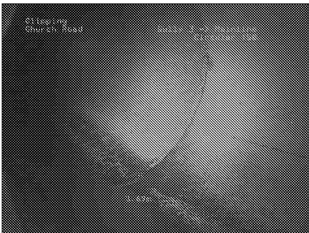
Photo: 46_5a 3.69m, Major connection without manhole
