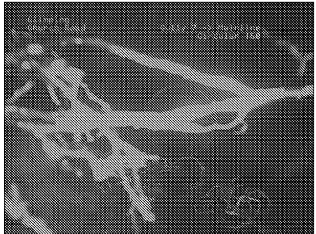
Photo: 83_3a 0.99m, Roots tap at joint
