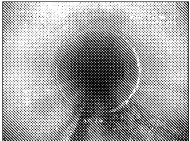
Photo: 127_12a 57.23m, Fine Roots at joint
