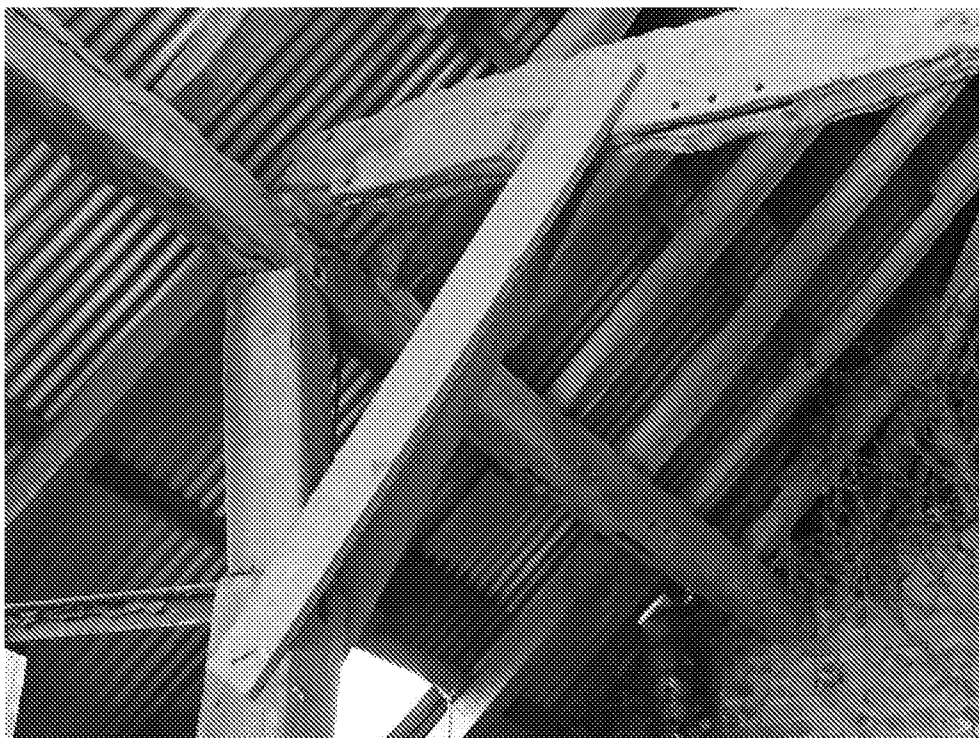
Photo of severed main post due to insertion of steel ties to west side aisle Note basic diagonal provided between main post and principal tie beam but diagonals missing between main post and eaves beam.
