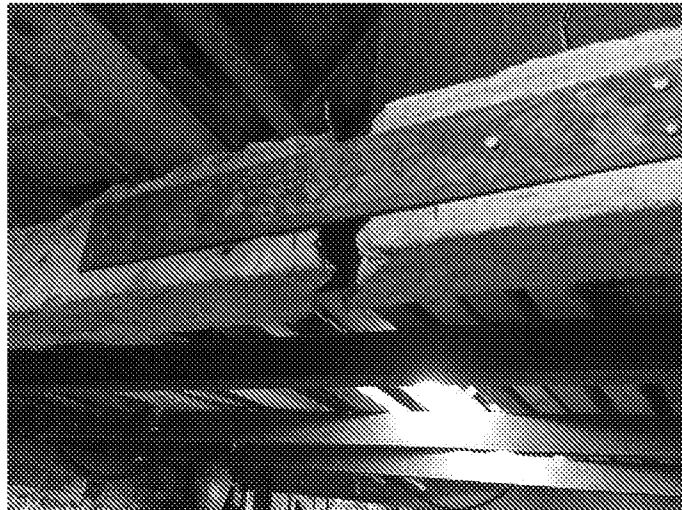
Photo of roof truss with failed principal tie beam.
