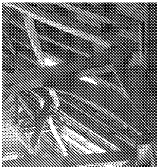
Photo showing timber decay to principal tie beam with loss of section causing joint to be ineffective.
