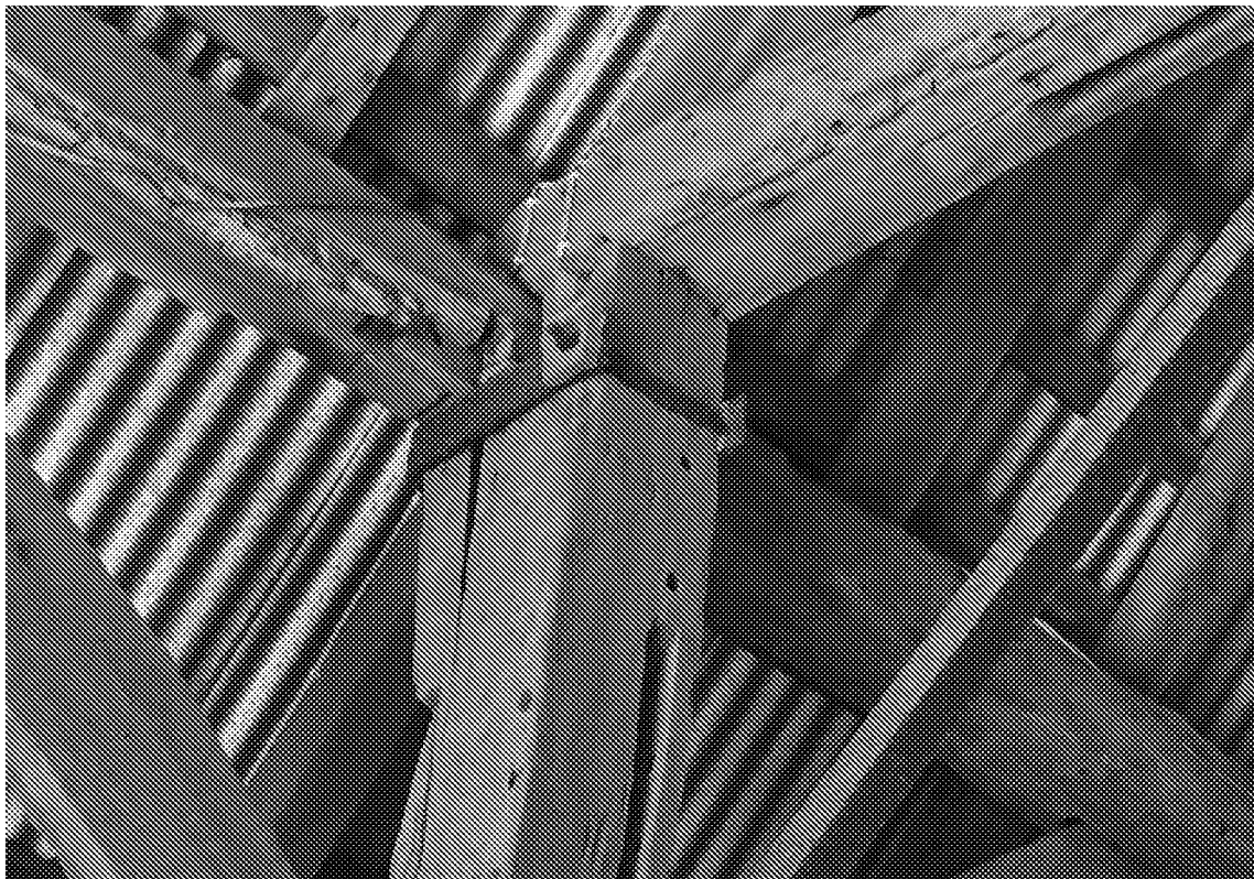
Photo of jowel sheared from post. Note missing diagonal brace between main post and principal tie beam.
