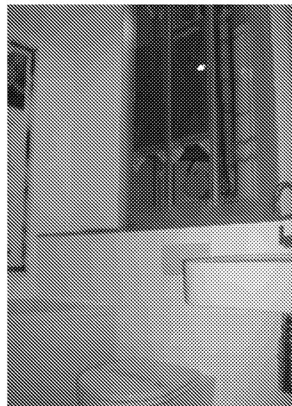
Figure 11: EcoPlay unit above WC
