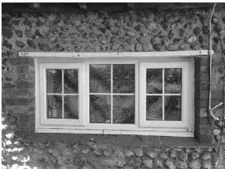
DSC03260: Inadequate timber lintel above triple casement failing Mill Thatch No2.
