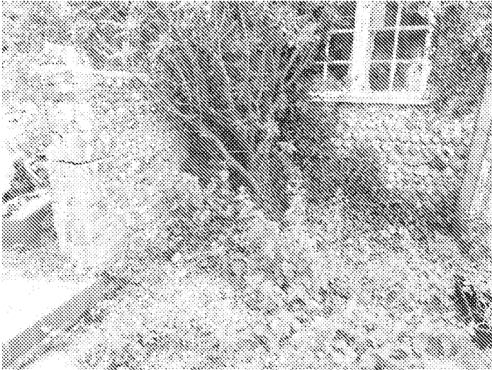
DSC02771: Evidence of cracking and settlement
