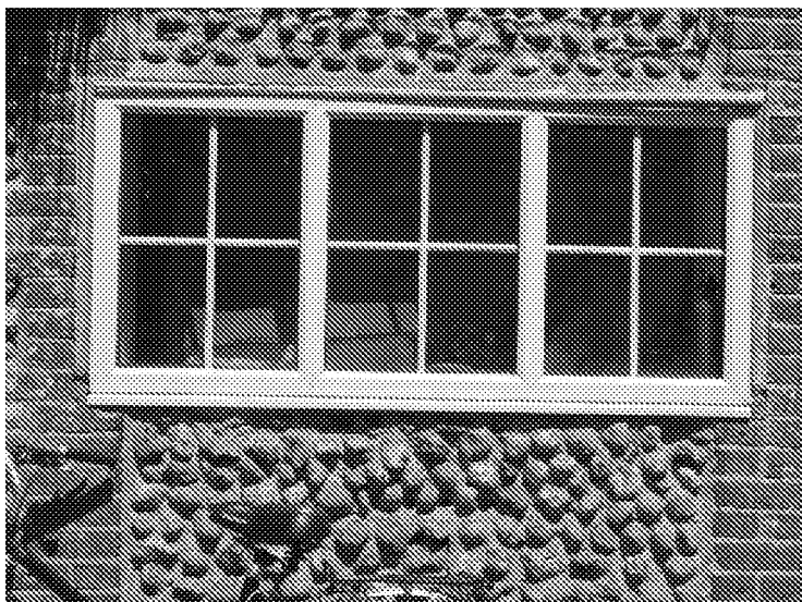
DSC03260 Enlarged opening encroaching upon brick dressings.
