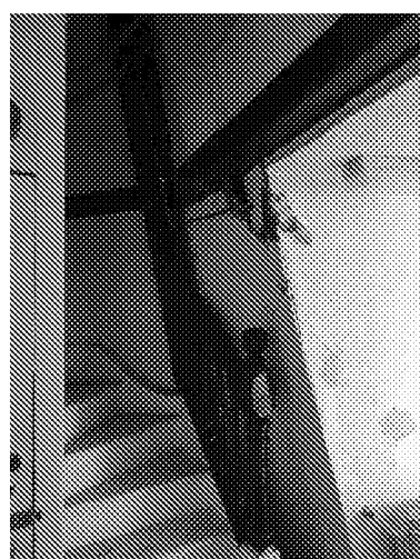
DSC02910 Inappropriate services and modern materials
