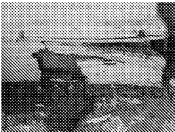
DSC02873 Dry rot in skirting
