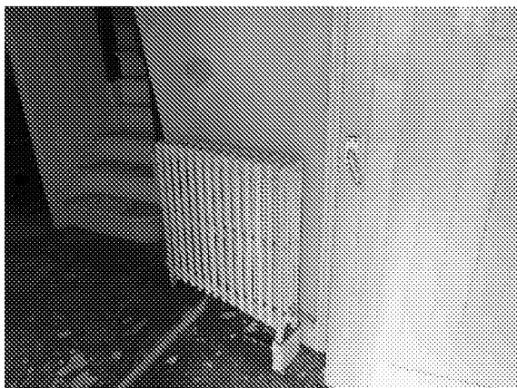
DSC02907 Cast iron radiator
