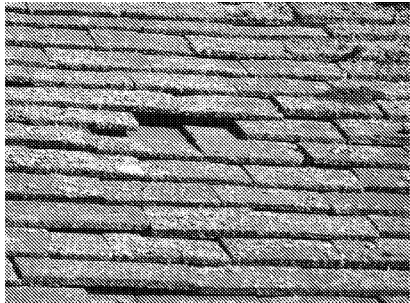
Gaps under missing roof tiles
