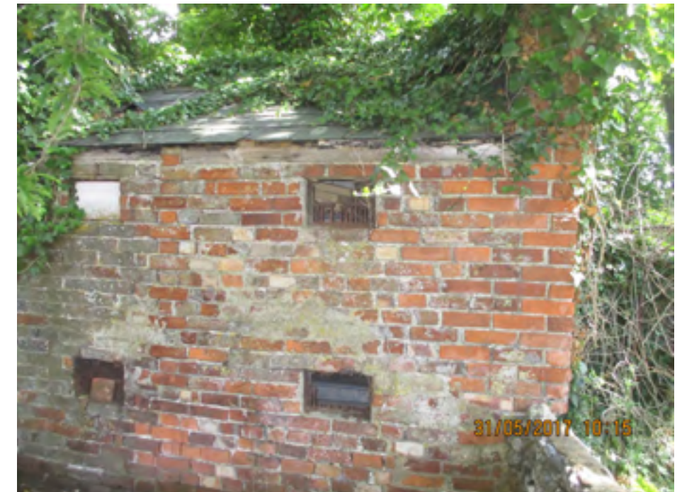
Erosion to pointing due to chronic water penetration. Structurally significant.
