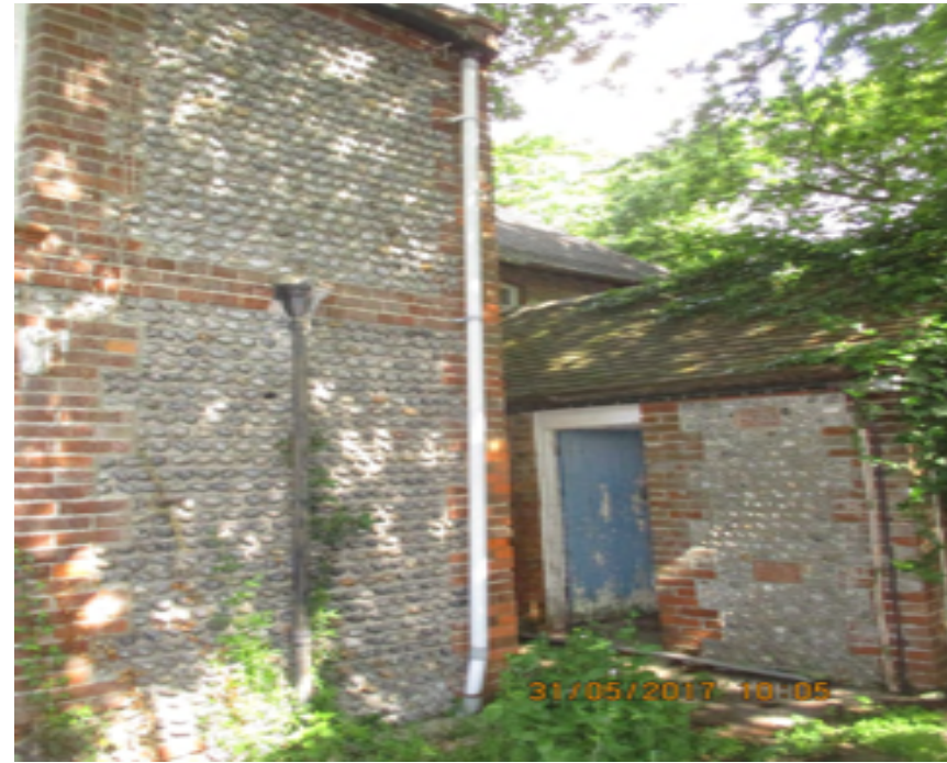
North end of east elevation; eaves gutter and rainwater downpipe replaced with narrow plastic rainwater goods, indicating failure of original rainwater goods.
