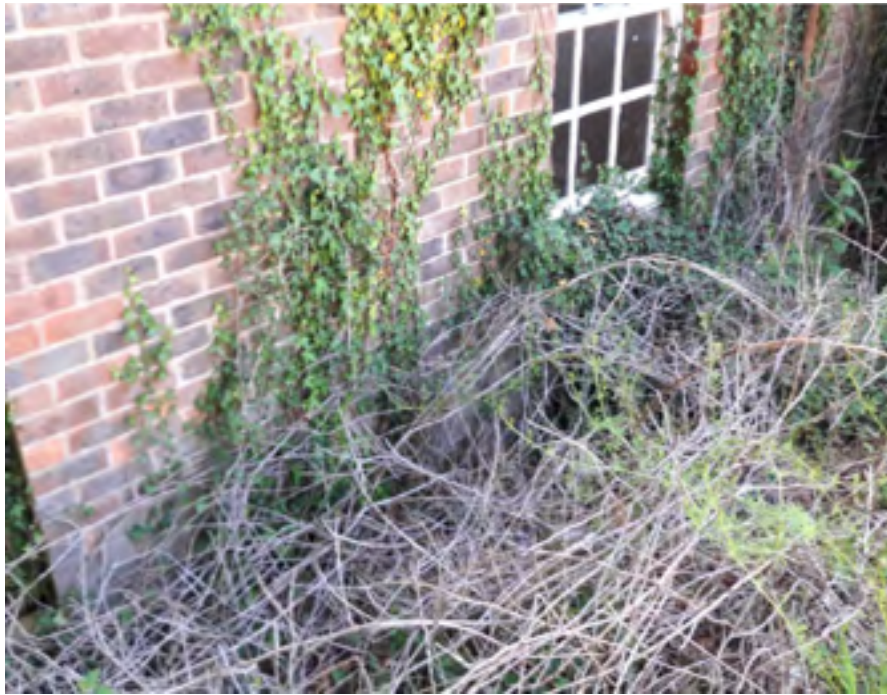
Chronic water penetration to structures beneath, providing conditions for damp and decay from roof to ground level. (see H&R report).
