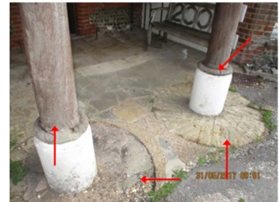
South elevation; showing base of timber posts, partially decayed by wet rot. They bore onto padstones or pillars beneath. Note previous repairs with concrete. These were very vulnerable to further decay and may no longer be structurally adequate. Also showing original composite mill stones forming paving at base
