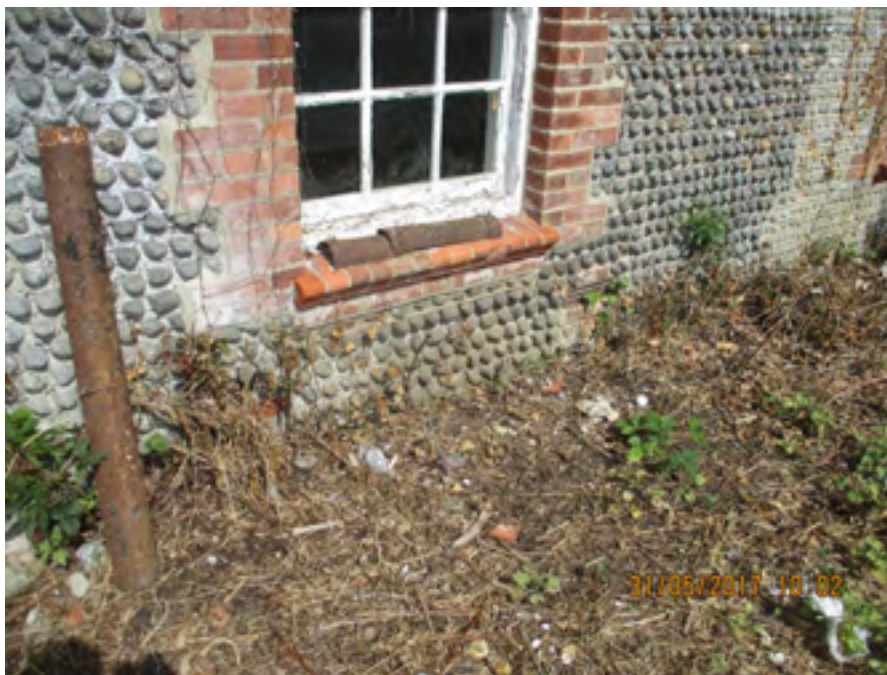
East elevation; ground levels above internal floor levels with ground and surface drainage encouraging water penetration to the base of walls and foundations, providing conditions for damp and decay. Also supplementary vents at the base of walls, presumably intended to serve sub-floor voids in the past and drainage gullies, blockage and overcharging.
