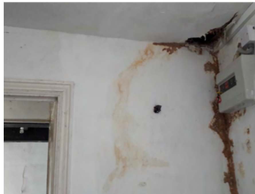
Chronic water penetration providing conditions for dry rot ( Serpula lacrymans ) infection and decay. Lintel over door of mill found to be structurally decayed.
