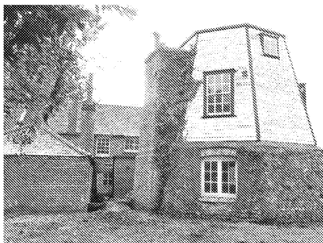
DSC02733 West Elevation Ivy growth to side of stack
