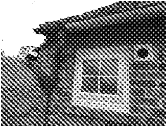
DSC03201: Low grade Upvc window & gutters, extractor
