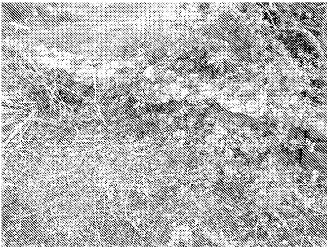
DSC032754: Dilapidated garden wall North of Mill Cottage
