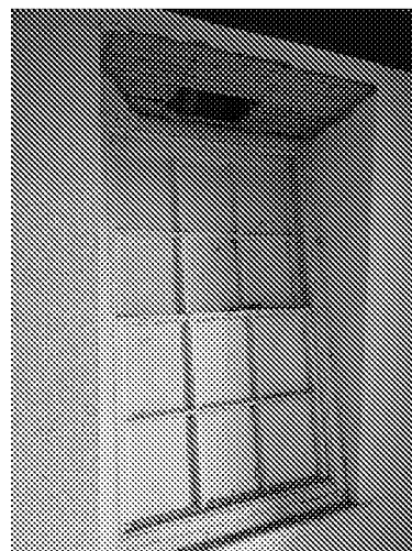
DSC02911 Boarded over window
