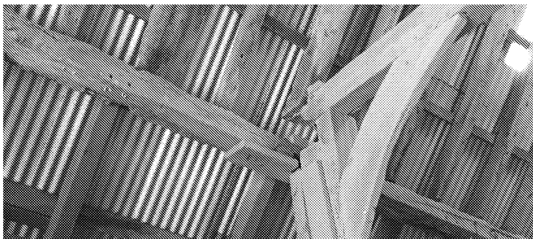
Photo of failed joint. Note diagonal braces missing between post and eaves beams
