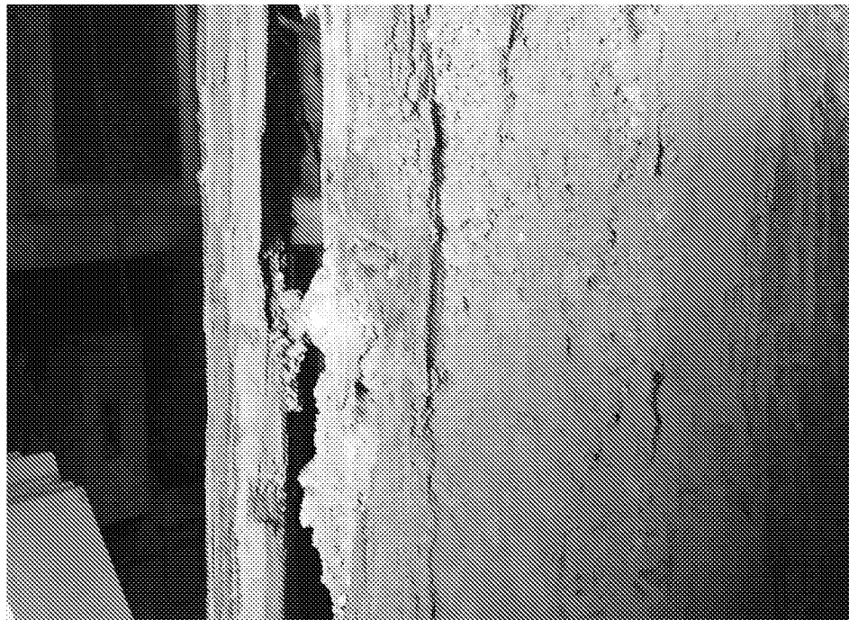
Photo of cement dust within cracks and crevices of a main post
