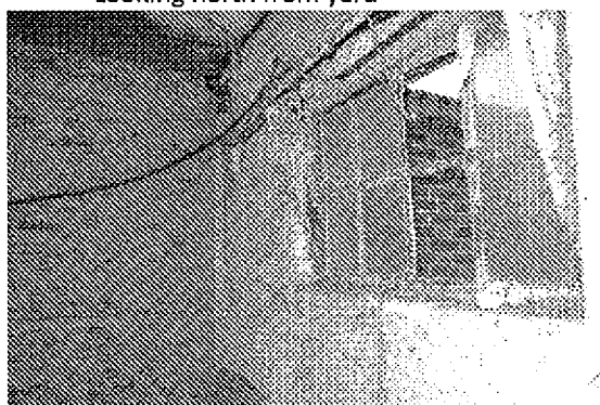
Missing window panes in stables, Building A
