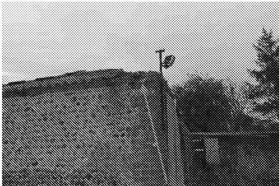
Damaged roof at south west corner
