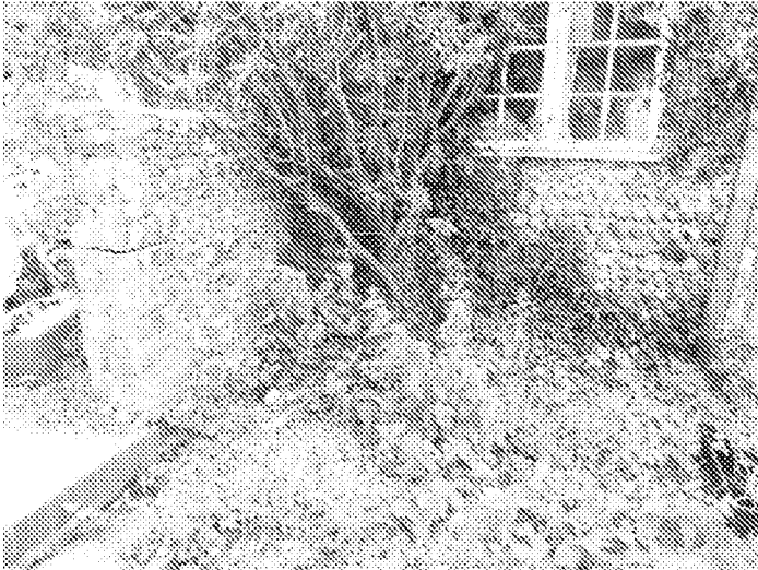
DSC02771: Evidence of cracking and settlement
