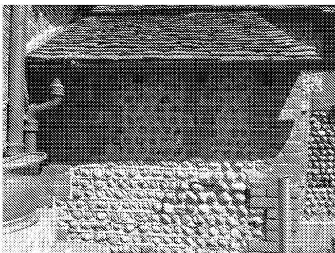
DSC03234: View of infilled former opening to lean-to and general degradation of mortar joints. Mill Cottage
