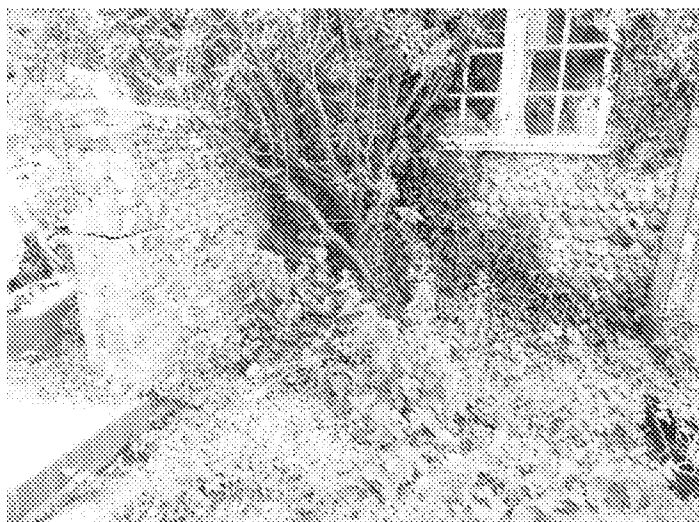
DSC02771: Evidence of cracking and settlement
