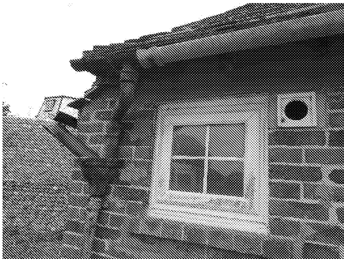
DSC03201: Low grade Upvc window & gutters, extractor
