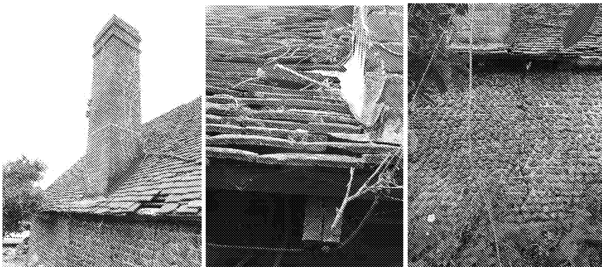
DSC02753 DSC03216, DSC03214: General defects including missing roof tiles, lead flashings & cracks to flintwork Mill Cottage, North Elevation.
