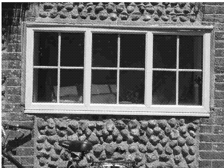
DSC03260 Enlarged opening encroaching upon brick dressings.
