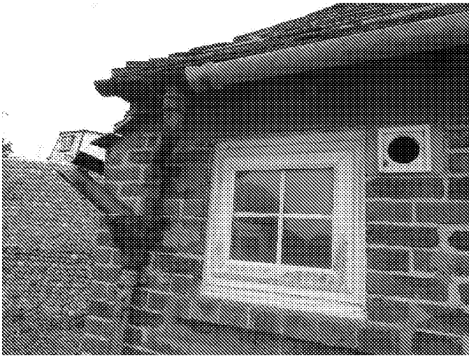
DSC03201: Low grade Upvc window & gutters, extractor
