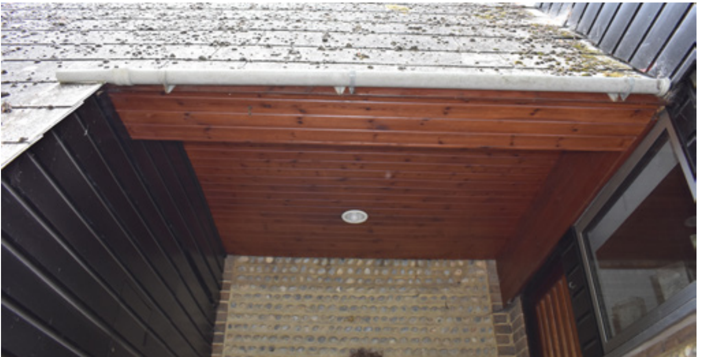
Photograph No. 04 - Connecting section between garage and main house, all materials sealing the wall and porch areas are aligned and tightly fitted into place against one another, no gaps are visible.
