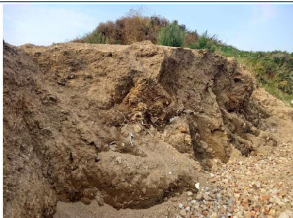
9. Soil stockpile which encroaches onto site from the south
