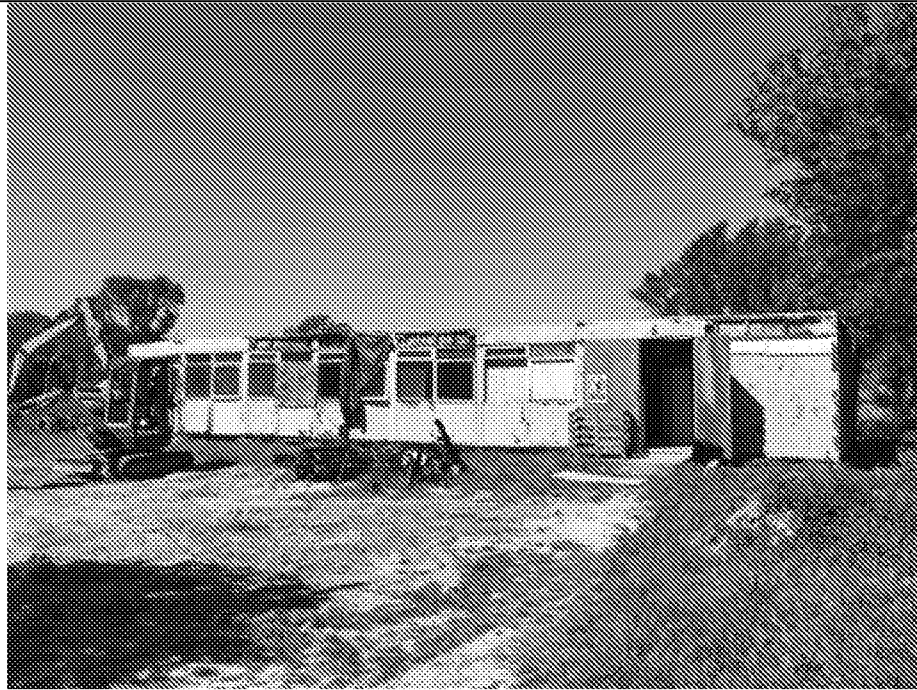
Building B4 – The Old School a prefabricated building in disrepair, currently used as a workshop and storage facility
