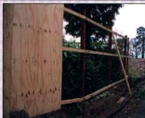
Board specification on secure wooden posts
