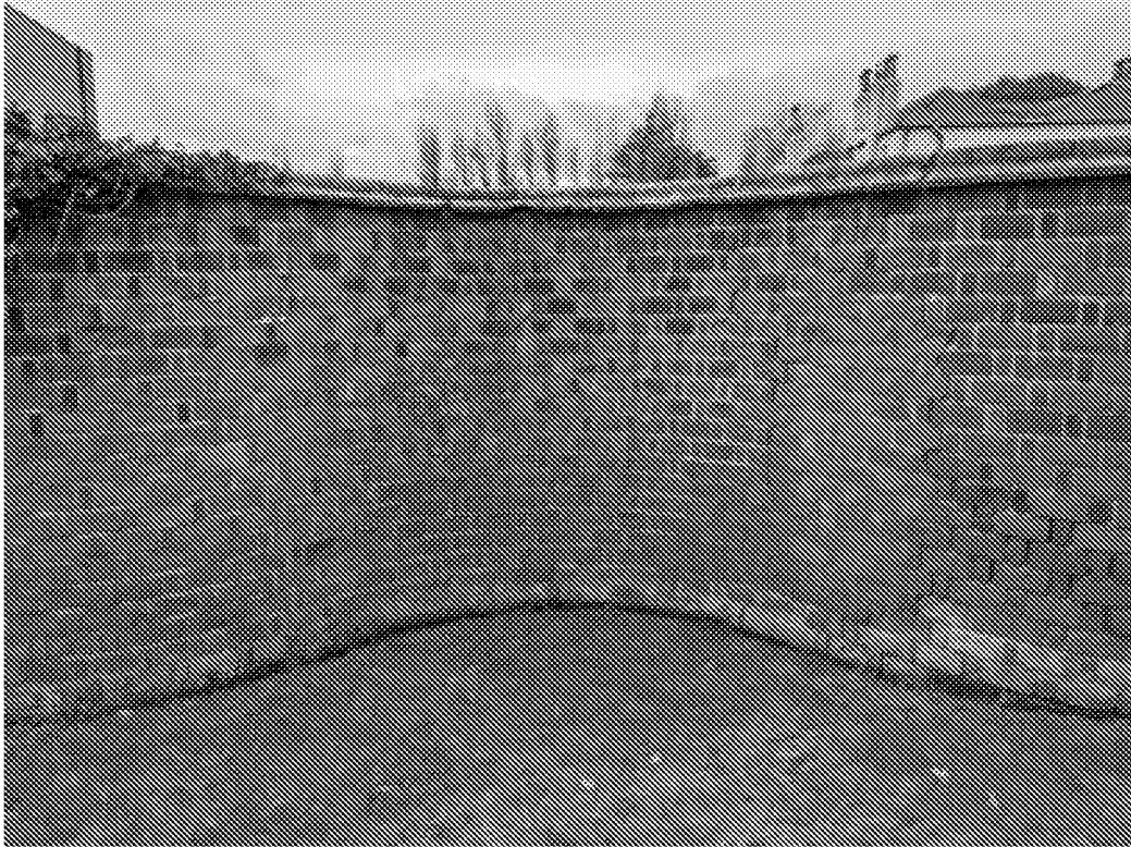
7 – Cracking on the northern face on section 6
