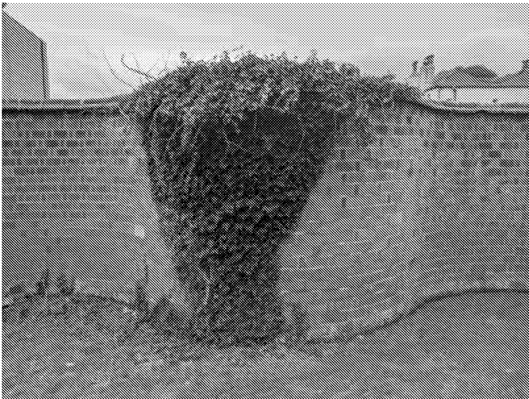
12 - Ivy growth on northern elevation of section 5
