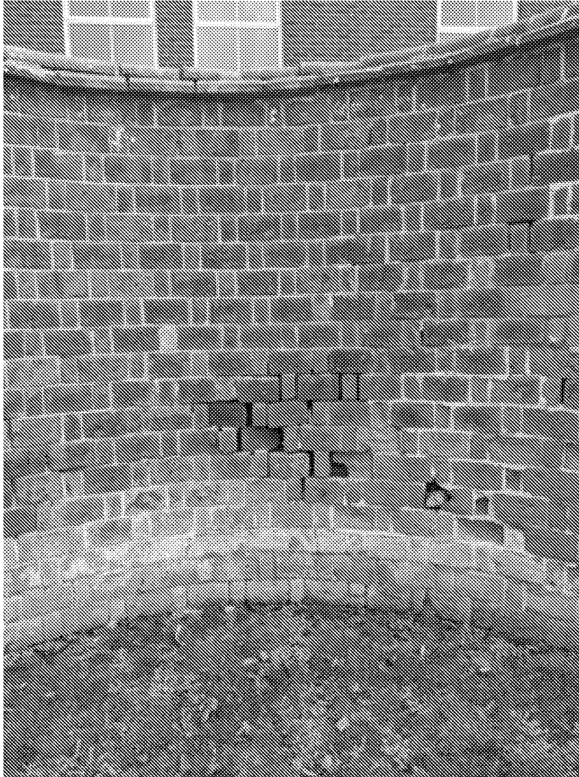
10 – Loss of mortar and bricks in southern face of section 9
