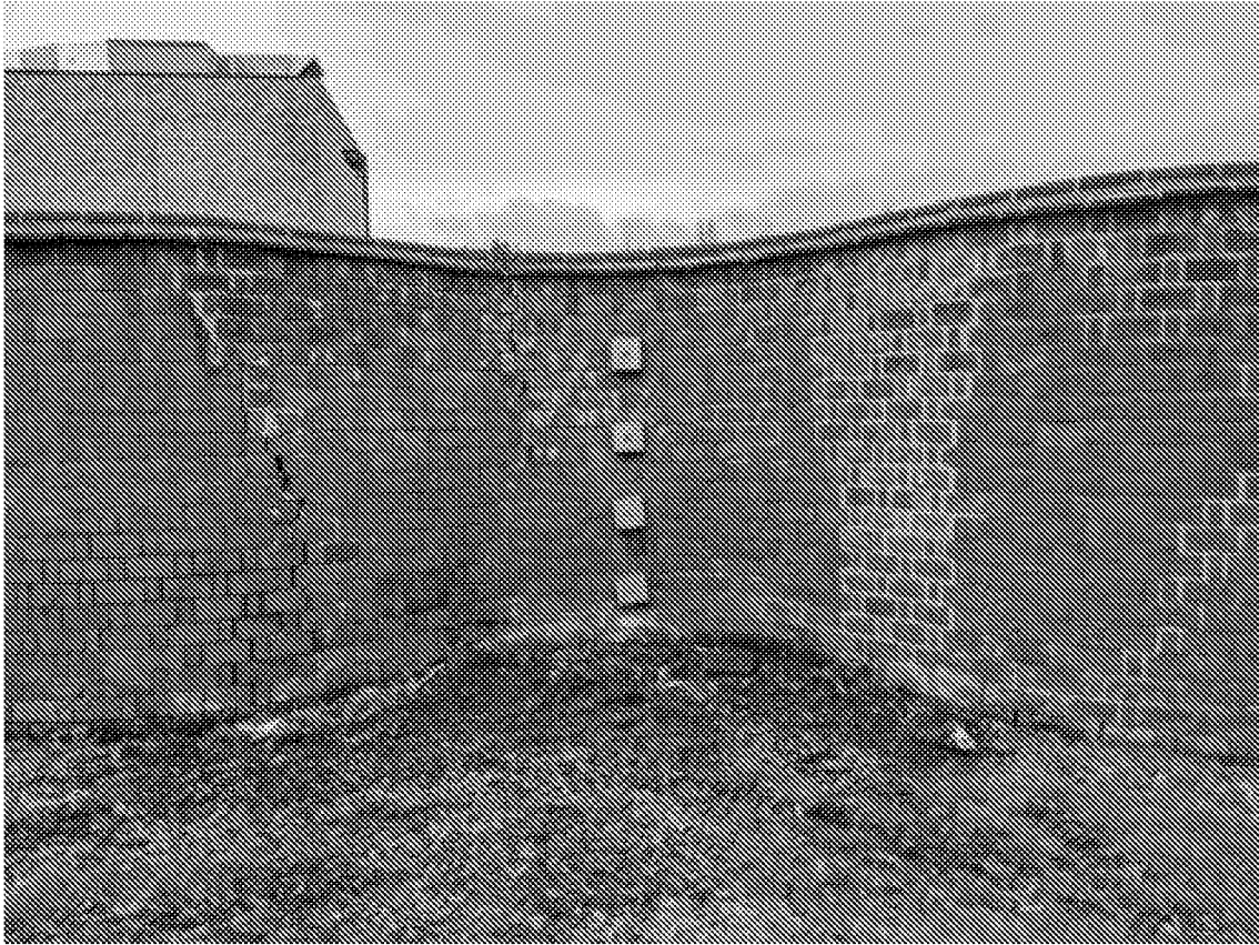
5 – Diagonal cracking on the northern face and evidence of historic repairs in section 2
