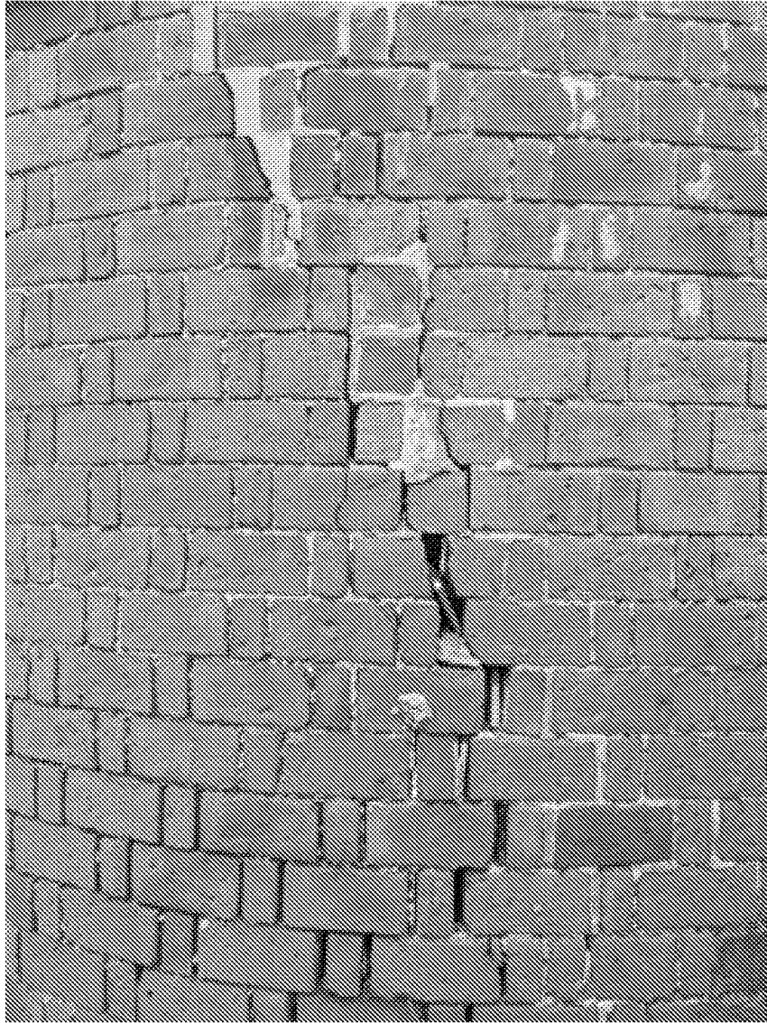
6 – Close-up of diagonal crack between sections 1 and 2 in photograph 5
