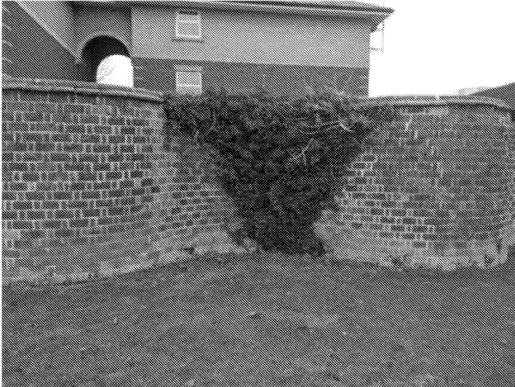
11 – Ivy growth on southern elevation of section 5
