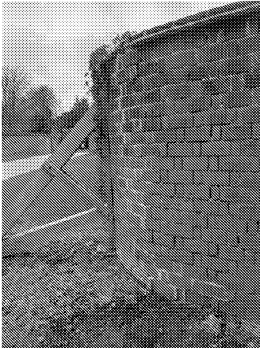
15 – Lean of section 2. Loss of mortar
