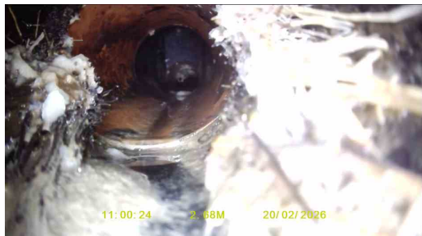
NEIGH MHX_353d599e-86f2-49f9-b787-79dede56729a_20260309_1 51525_153.jpg, 00:00:38, 2.68 m Roots, mass at joint, 15% cross-sectional area loss
