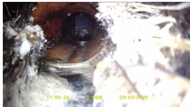
NEIGH MHX_98e14b0c-5078-47af-9d1d-c4fecb05a7b2_20260309_1 51545_215.jpg, 00:00:38, 2.68 m Material changes to polyvinyl chloride
