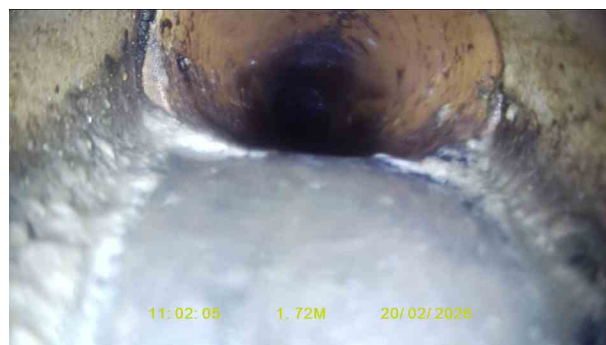
MH1X_87134125-87be-4706-885c-f264c308d8d2_20260309_1 152055_841.jpg, 00:00:25, 1.72 m Attached deposits, encrustation at joint from 4 o'clock to 8 o'clock, 20% cross-sectional area loss
