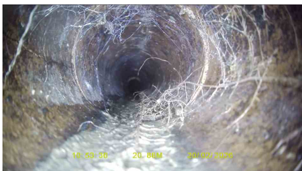
UNKNOWNX_01b833da-1af9-40f4-82e7-59b4f9813641_20260309_150915_546.jpg, 00:02:26, 20.86 m Roots, fine at joint
