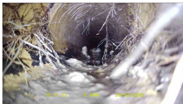
UNKNOWNX_96da4866-93d6-40c9-935e-2d70b43f70ff_2026 0309_150543_965.jpg, 00:00:22, 0.48 m Roots, fine at joint
