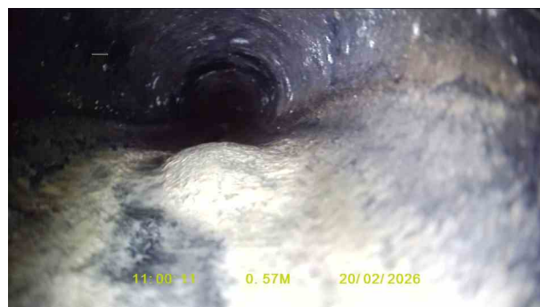
NEIGH MHX_1eb83b89-b91b-4ed7-9275-ab4ff6b04c27_20260309_1 51341_728.jpg, 00:00:26, 0.57 m Deformed drain or sewer, 10%
