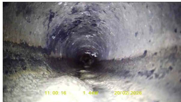
NEIGH MHX_d0afc9db-651f-46b0-b605-d325d48d1f4a_20260309_15 1421_041.jpg, 00:00:30, 1.44 m Deformed drain or sewer, 5%
