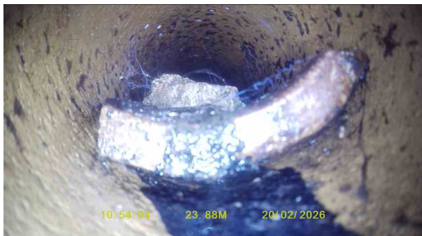
UNKNOWNX_ee8bb757-b272-4aac-8351-86a90515e417_20260309_151006_881.jpg, 00:02:53, 23.88 m Settled deposits, coarse, 50% cross-sectional area loss
