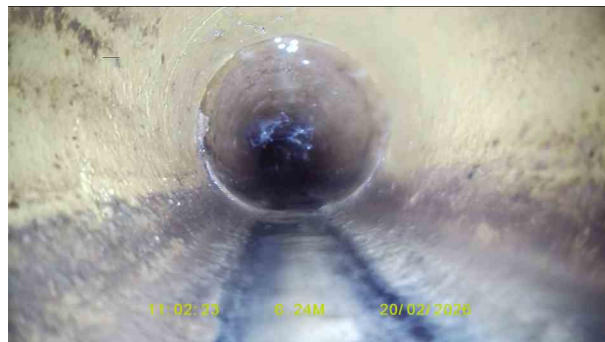
MH1X_b7e21036-a785-4a45-a376-16d1e7c6e280_20260309_152237_006.jpg, 00:00:43, 6.24 m Crack, circumferential at joint from 8 o'clock to 12 o'clock
