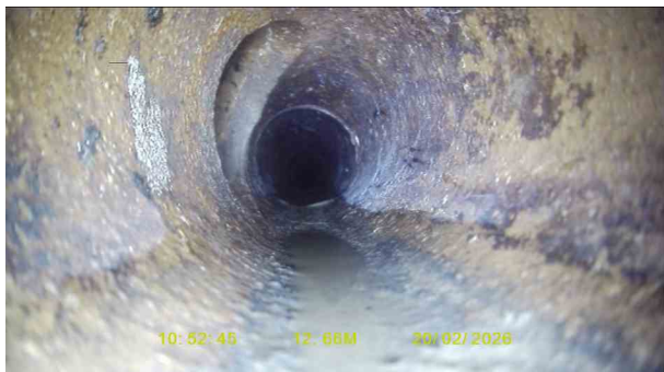
UNKNOWNX_2e3493d6-f1b9-4e51-ab53-bfb978736c69_20260309_150812_778.jpg, 00:01:35, 12.66 m Junction at 9 o'clock, diameter: 100mm
