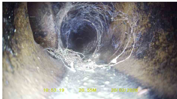
UNKNOWNX_8ab6bb7f-afb5-46a2-97ad-c9e97d645cf4_20260309_150852_478.jpg, 00:02:09, 20.55 m Defective junction, damaged at 9 o'clock, diameter: 100mm, CRACKED & ROOT INFILTRATED
