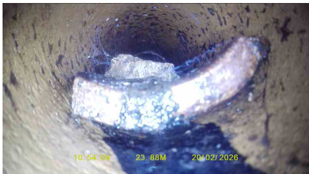
UNKNOWNX_ee8bb757-b272-4aac-8351-86a90515e417_20260309_151006_881.jpg, 00:02:53, 23.88 m Settled deposits, coarse, 50% cross-sectional area loss
