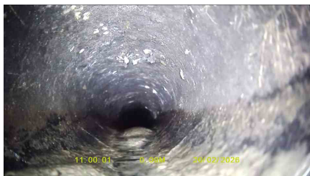
NEIGH MHX_cbc27641-9414-4772-a36f-8aa1791142d9_20260309_1 51317_993.jpg, 00:00:16, 0.09 m Deformed drain or sewer, 10%
