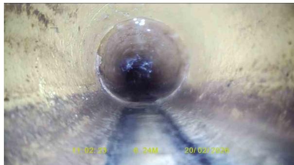
MH1X_b7e21036-a785-4a45-a376-16d1e7c6e280_20260309_152237_006.jpg, 00:00:43, 6.24 m Crack, circumferential at joint from 8 o'clock to 12 o'clock
