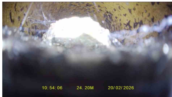
UNKNOWNX_c0d73047-4b10-4f56-afd4-2bcc42f0deb9_20260309_151038_481.jpg, 00:02:56, 24.20 m Survey abandoned, S/A - UNABLE TO PASS DEBRIS
