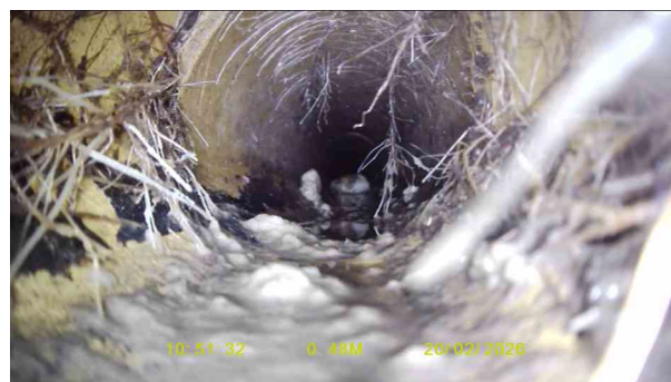
UNKNOWNX_96da4866-93d6-40c9-935e-2d70b43f70ff_2026 0309_150543_965.jpg, 00:00:22, 0.48 m Roots, fine at joint
