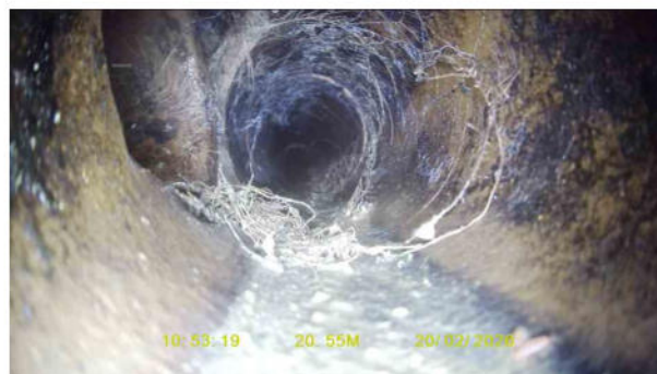
UNKNOWNX_8ab6bb7f-afb5-46a2-97ad-c9e97d645cf4_20260309_150852_178.jpg, 00:02:09, 20.55 m Defective junction, damaged at 9 o'clock, diameter: 100mm, CRACKED & ROOT INFILTRATED
