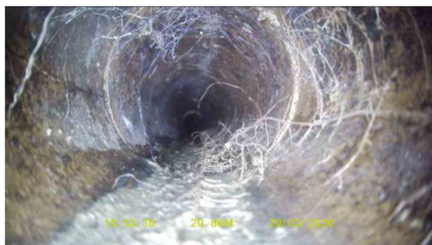
UNKNOWNX_01b833da-1af9-40f1-82e7-59b1f9813641_20260309_150915_546.jpg, 00:02:26, 20.86 m Roots, fine at joint
