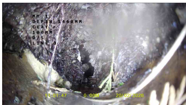
MH1X_5f86450e-be3e-4e2f-bdc8-18a30d40e5f7_20260309_1 52026_783.jpg, 00:00:07, 0.02 m Roots, mass at joint, 80% cross-sectional area loss
