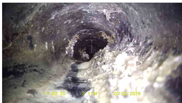
NEIGH MHX_8c17c4af-3b21-4ba9-a9eb-daf083b01de2_20260309_1 51444_714.jpg, 00:00:34, 2.11 m Deformed drain or sewer, 20%
