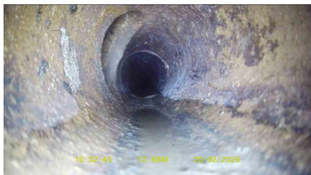
UNKNOWNX_2e3493d6-f1b9-4e51-ab53-bfb978736c69_20260309_150812_778.jpg, 00:01:35, 12.66 m Junction at 9 o'clock, diameter: 100mm
