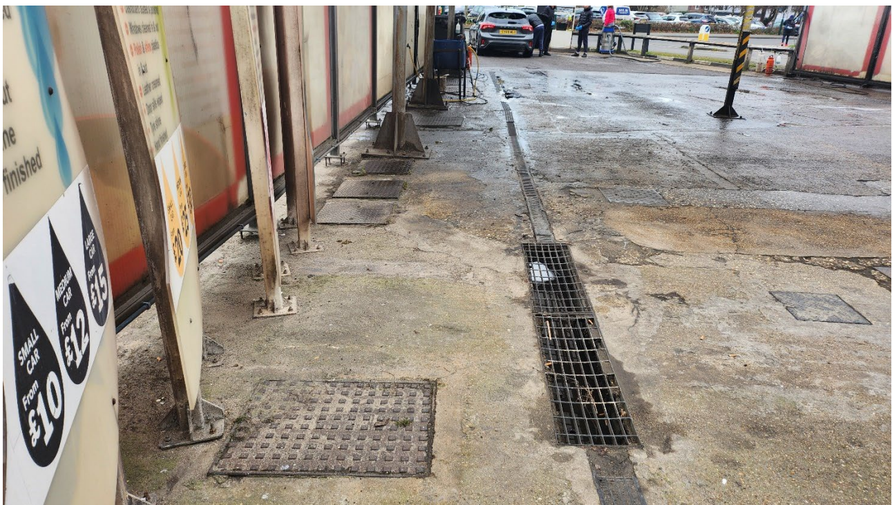
Plate 10 View of inspection covers located along the eastern site boundary, likely presence of drainage/interceptors
