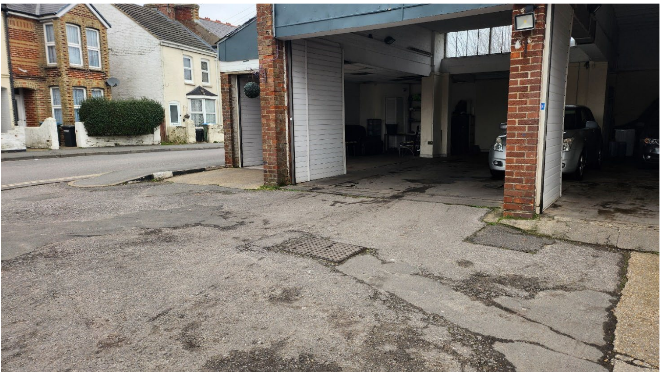
Plate 6 View of inspection chamber in north of site, possible presence of UST
