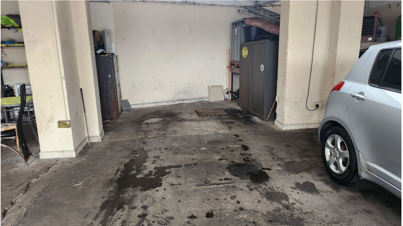
Plate 5 Inspection chamber located inside the building in the north of the site, possibly indication of presence of UST
