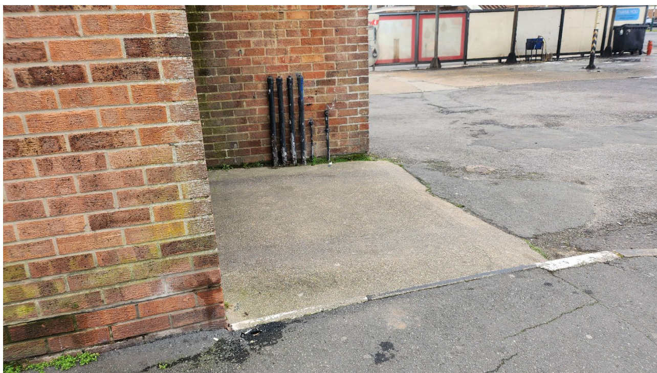
Plate 4 View of breather pipes located adjacent to the buildings in the north of the site
