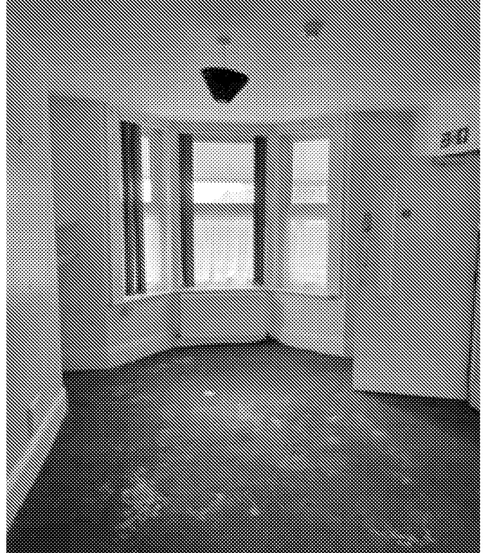
Milton Lodge at ground floor, showing signs of disrepair
