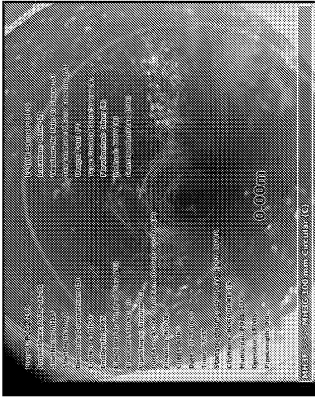
20230601-073850-snap0000.jpg, 00:00:00, 0.00 m Start node, manhole, reference: MH3F
