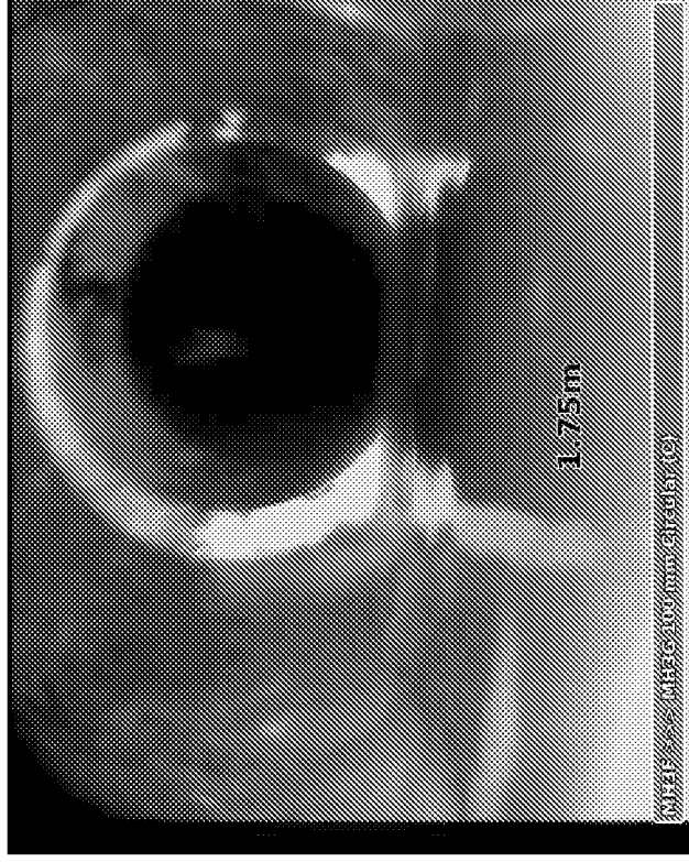
MH3FX_3af06dc0-f12a-4d8a-80fb-3cc04be7210f_20230614_1 01252_116.jpg, 00:00:38, 1.75 m Other obstacles in invert from 12 o'clock to 12 o'clock, 20%
