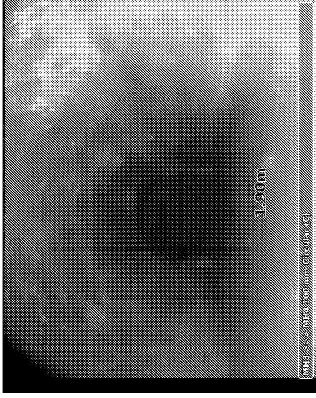
MH3X_c82d175f-90ef-4a86-b861-dc71ca4787b6_20230614_10 2256_091.jpg, 00:00:23, 1.90 m Water level, 20% of the vertical dimension
