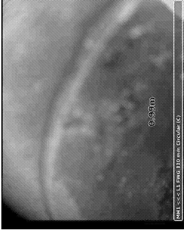
20230601-051525-snap0001.jpg, 00:00:21, 0.99 m Finish node, gully, reference: L1 FWG
