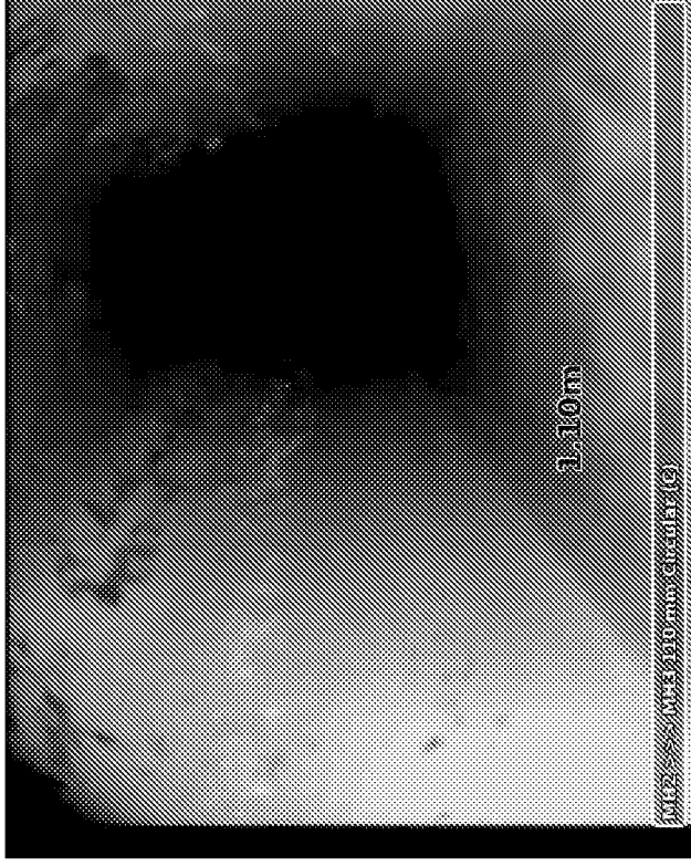
MH2X_0630e854-a7c9-4f85-9eaf-0ea1f6178117_20230614_09 4433_834.jpg, 00:00:21, 1.46 m Settled deposits, other, 10% cross-sectional area loss, start
