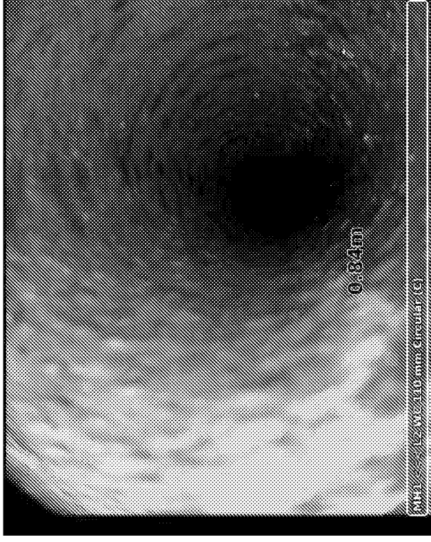
20230601-052126-snap0001.jpg, 00:00:21, 0.84 m Material changes to cast iron
