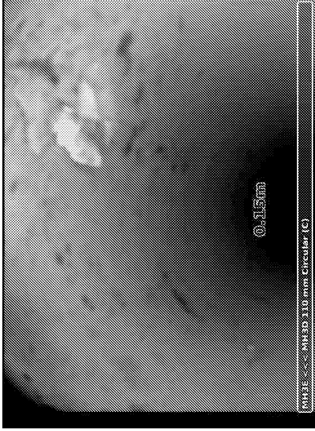
MH3DX_12079f60-eeef-47b3-9e33-27eedd567b02_20230615_143944_949.jpg, 00:00:03, 0.20 m Hole in drain or sewer at 1 o'clock
