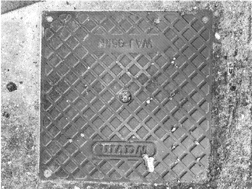
Unable to remove screws on MH3D
