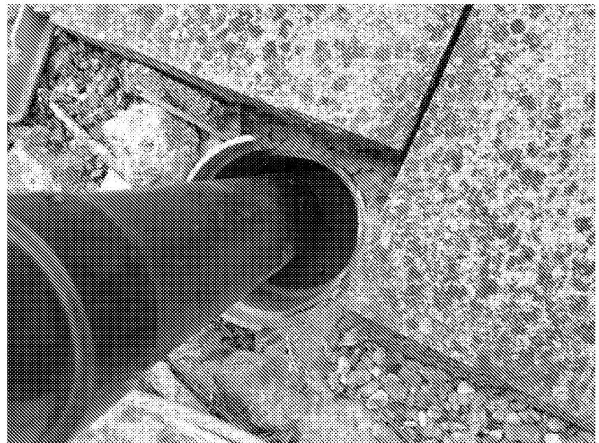
RWP1 rest bend broken
