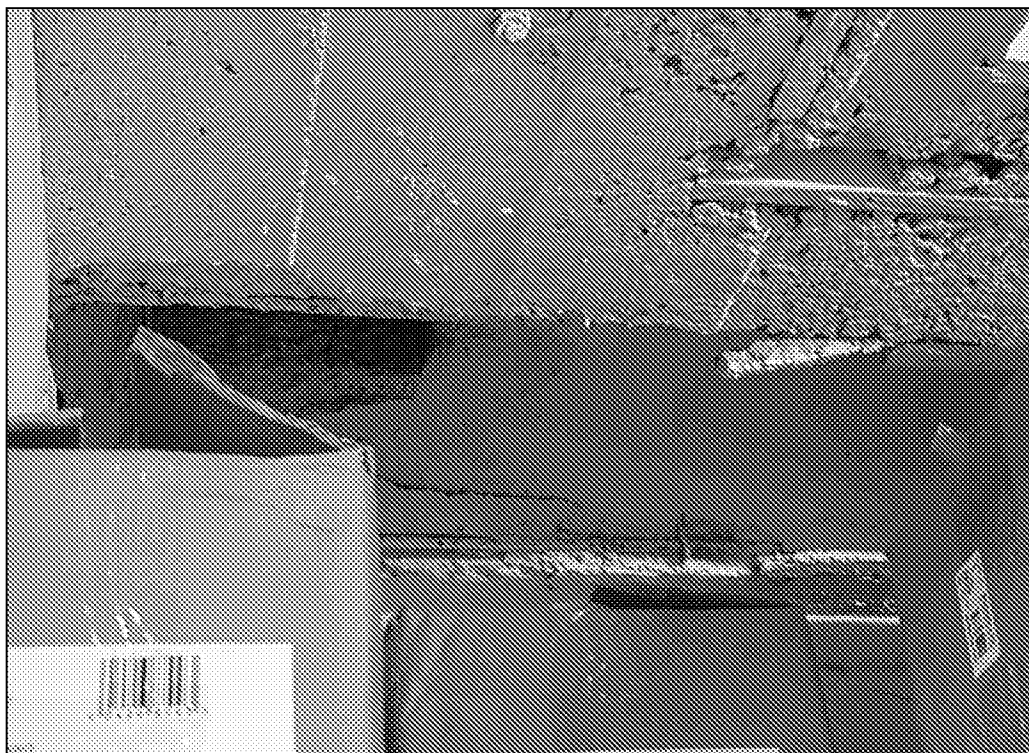
Photograph 3 – Severed steel reinforcement
