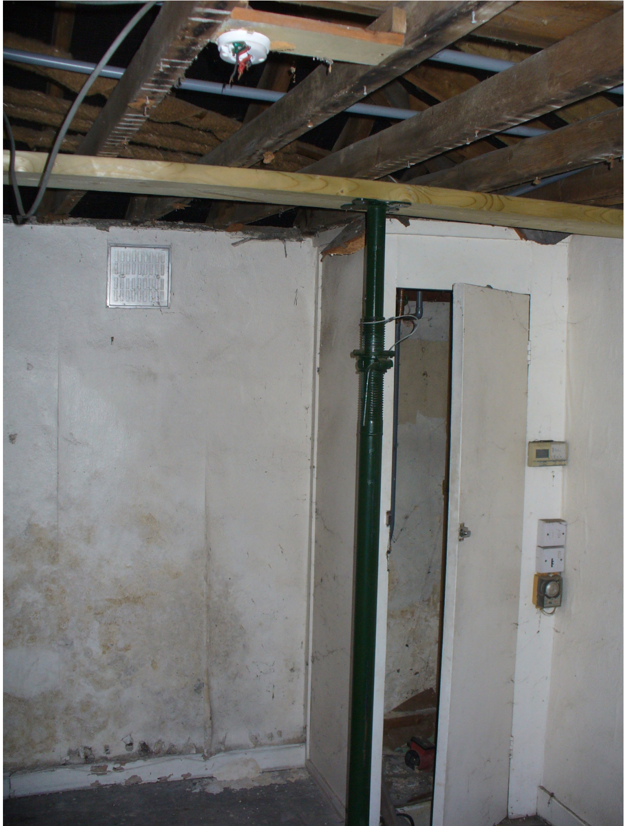
69 Upper Bognor Road Airing cupboard in corner of bedroom
