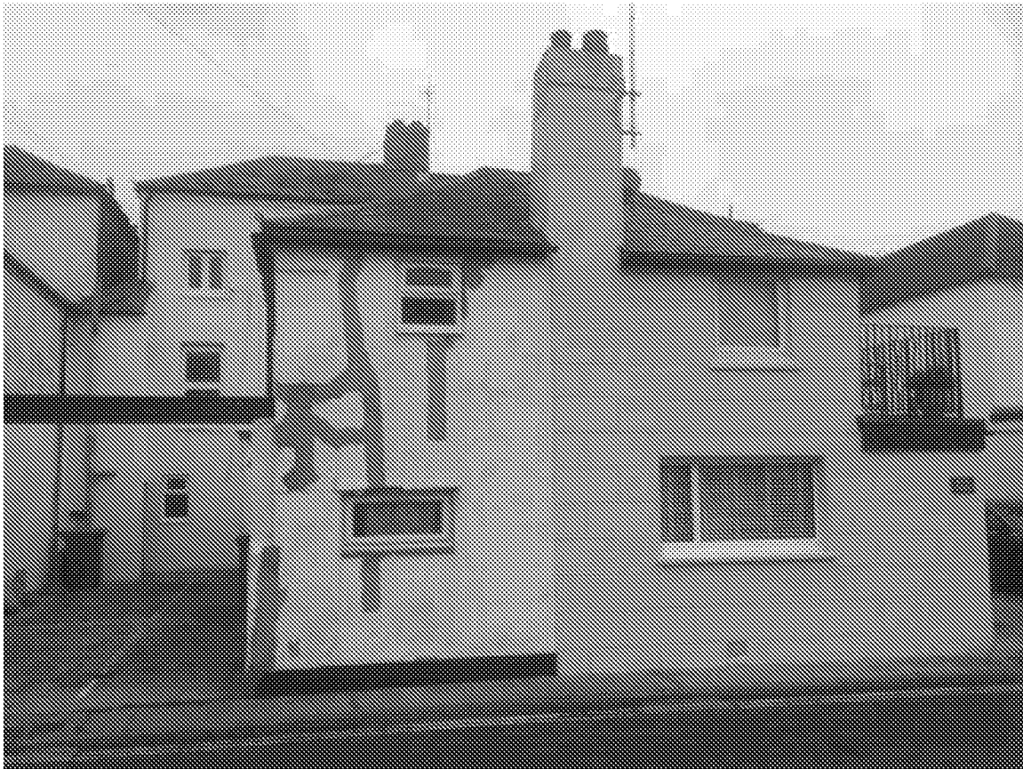
Rear of 9b Waterloo Square (left), note neighbouring approved extension and UPVC
