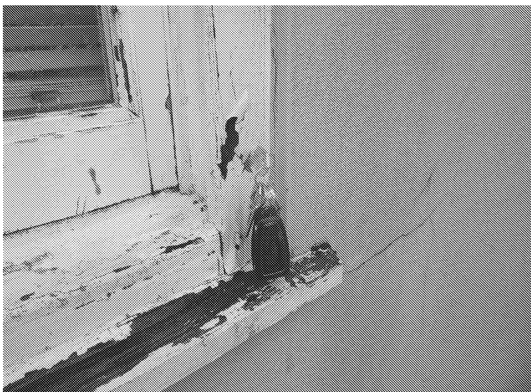
8.2 Existing window deterioration II
