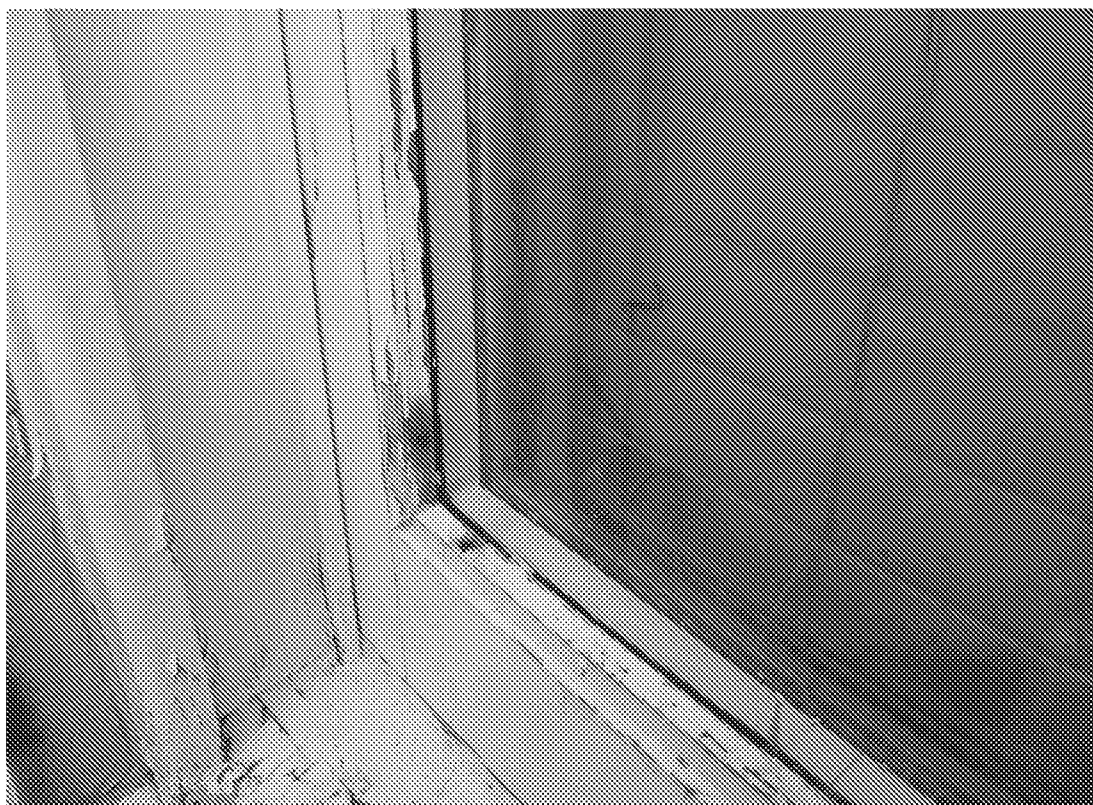
8.1 Typical Existing window deterioration I
