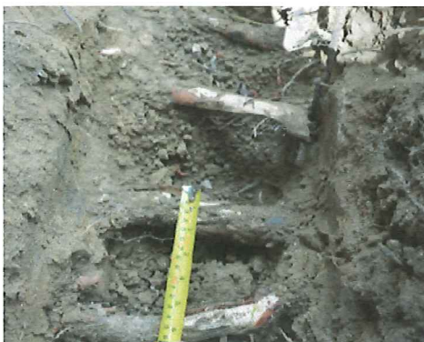
Trench along curved kerb edge. Roots up to 50mm at 300mm depth
