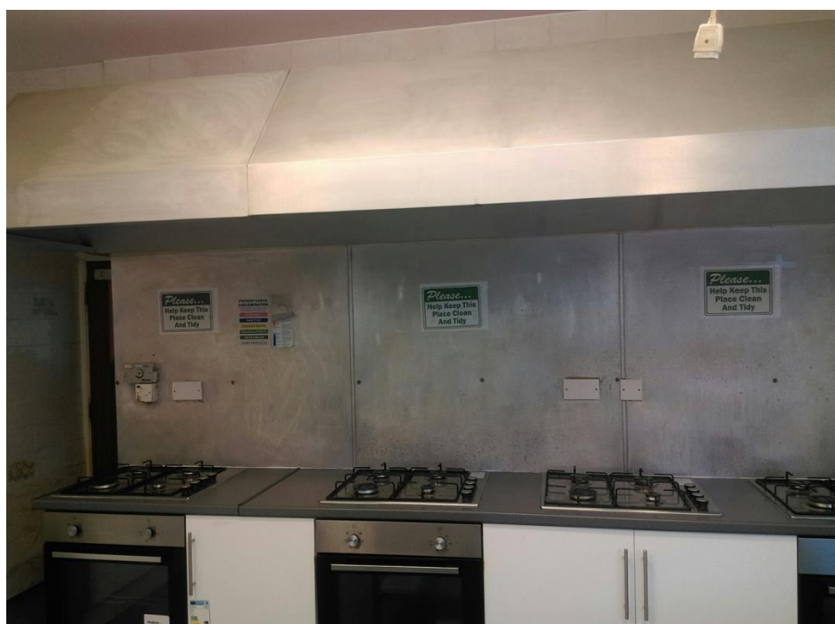
Photo 2 – view of cooking facilities
