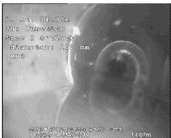
190521_1123A-Survey.jpg, 00:01:00, 14.07 m Junction, at 03 o'clock, diameter: 100 mm
