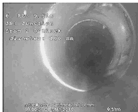
190521_1000A-Survey.jpg, 00:01:10, 9.51 m Junction, at 02 o'clock, diameter: 100 mm
