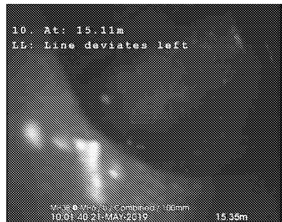
190521_1001D-Survey.jpg, 00:01:41, 15.37 m Line deviates left
