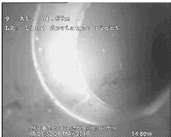
190521_1001C-Survey.jpg, 00:01:38, 14.81 m Line deviates right
