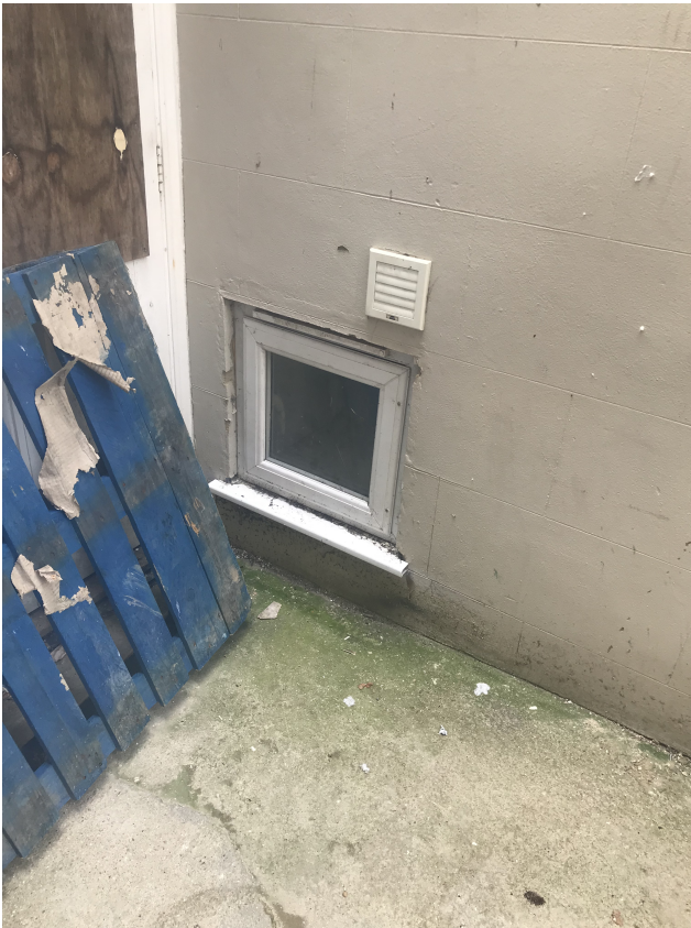
UPVC flat 1 window to be replaced
